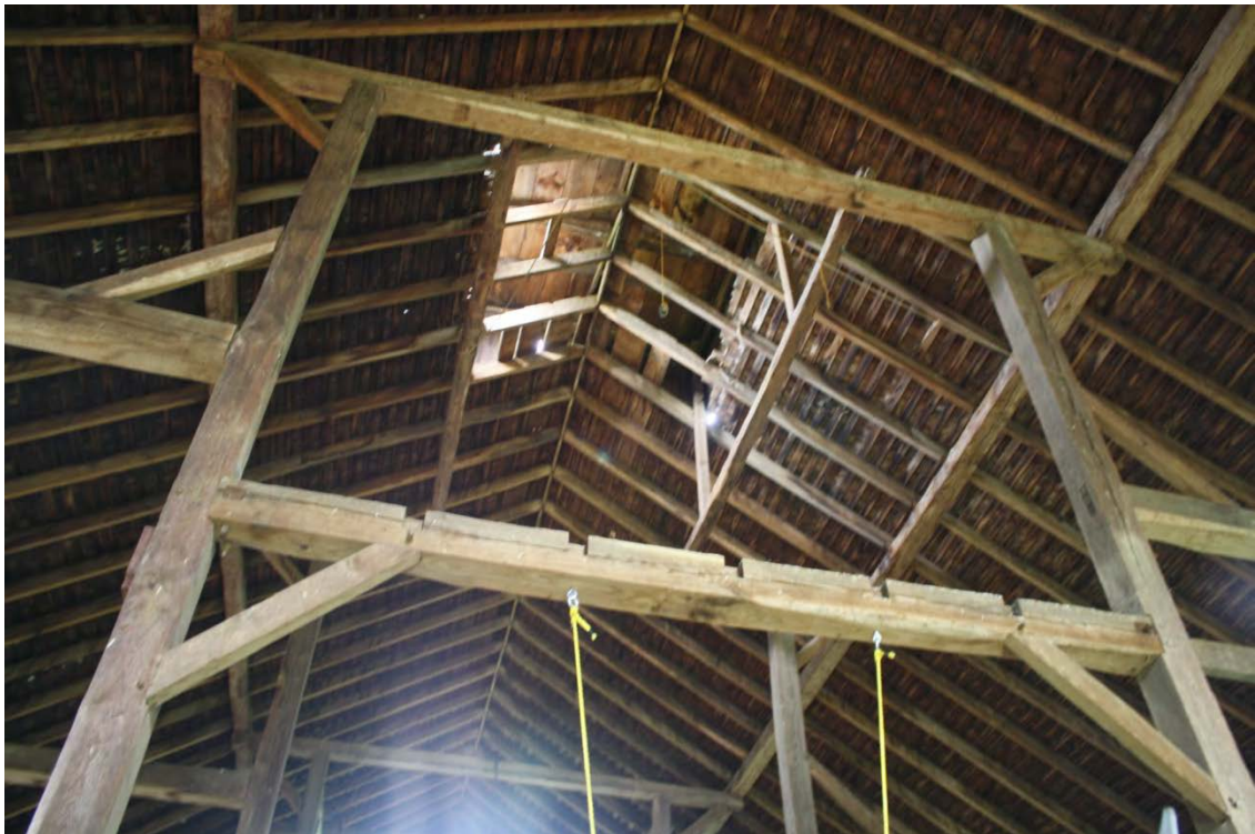
12. Interior view of Barn I main level, camera facing west, with cantilevered top tie girls supporting purlin plates.
