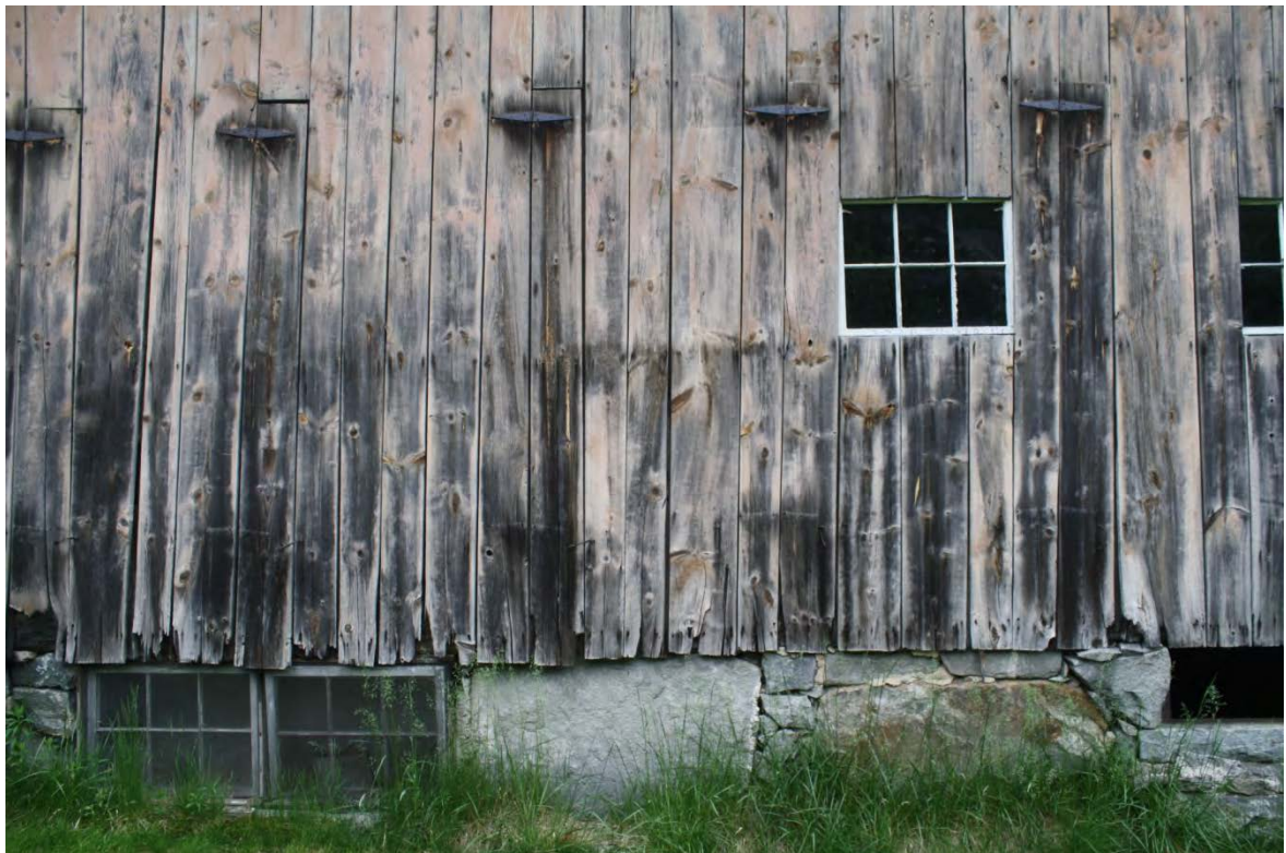
16. North detail view of Barn II, camera facing south; showing stone foundation and tobacco shed venting.
