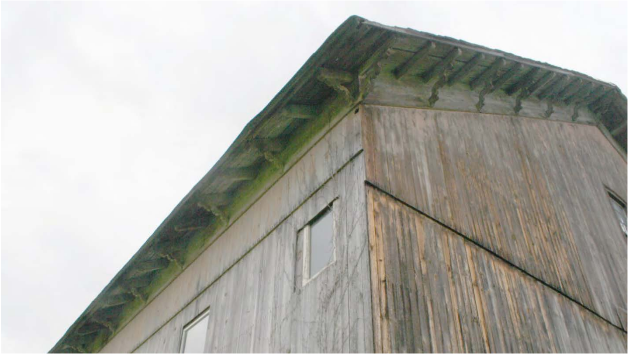
9. Northwest view of Barn I eave and rake details, camera facing southeast.
