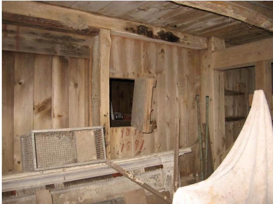
20. Interior view of Barn I lower level, showing openings between carriage bay and horse stalls, camera facing northeast.
