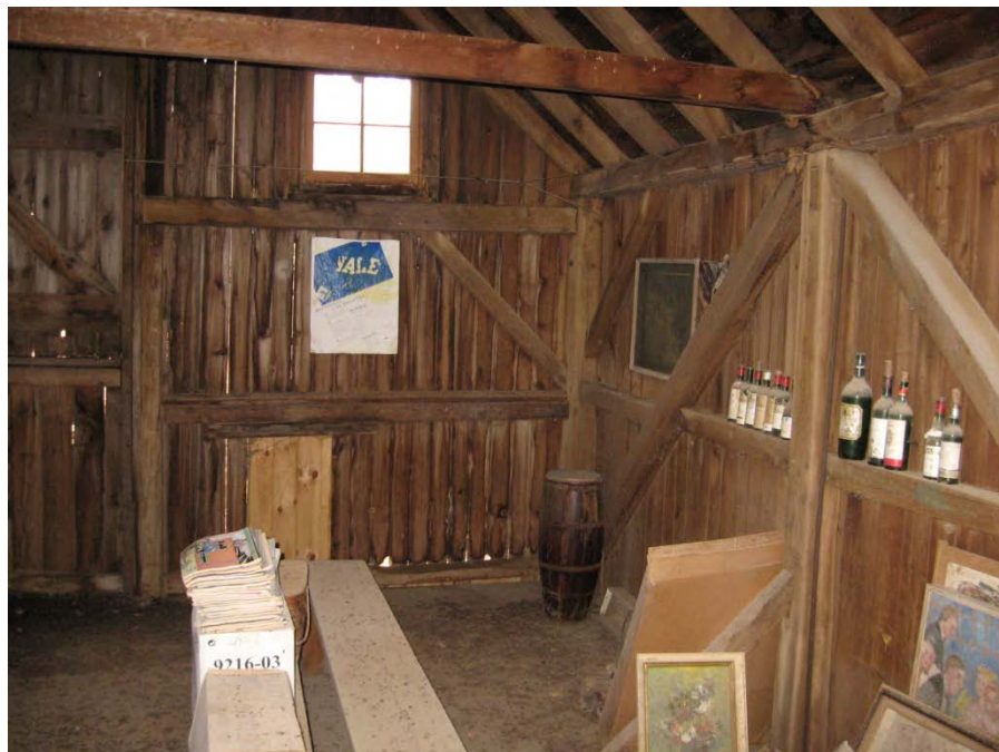
15. Interior view of Barn I second floor level, showing framing detail, camera facing southeast. Note location of removed tie-girt and framing over south bay opening at right.
