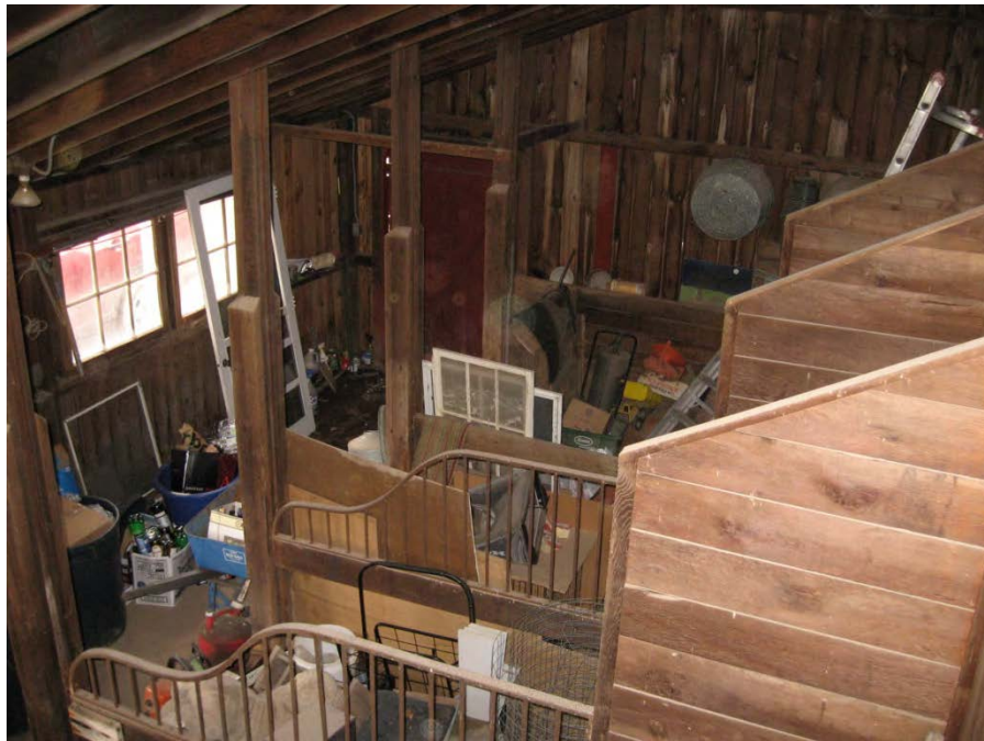
17. Interior view of Barn I north addition, showing horse stalls, camera facing northeast. Note the iron stanchions.
