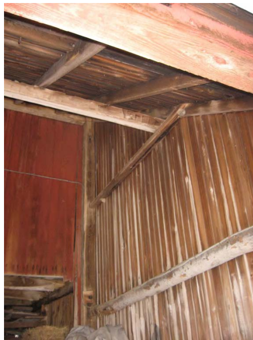
21. Interior view of Barn I south addition, showing recycled framing, camera facing northeast.
