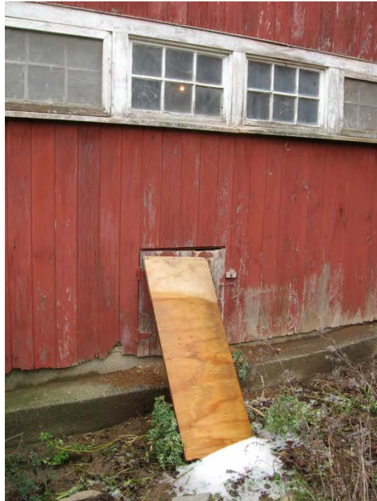
14. South elevation of Barn I, camera facing northeast. Detail of hopper windows and chicken run door.
