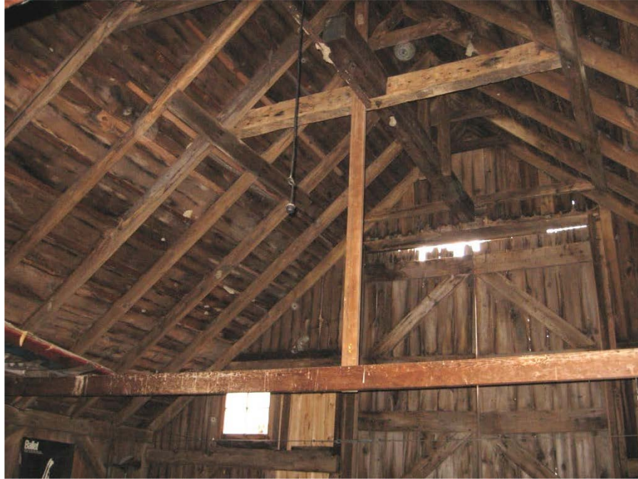
16. Interior view of Barn I second floor level, showing framing detail of hay track, camera facing northeast. Note replacement support framing and hay door at rear.
