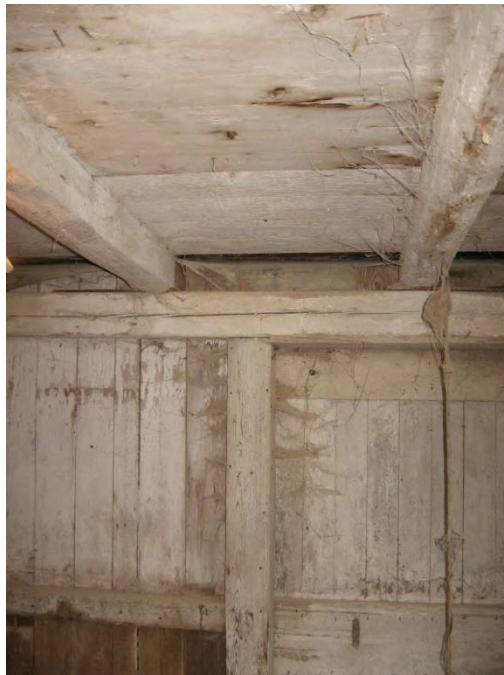
19. Interior view of Barn I lower level, showing whitewashed walls and ceiling, camera facing east.
