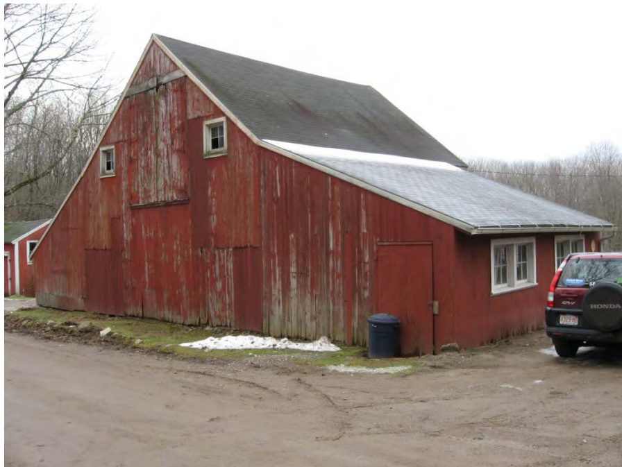
11. East and north elevations of Barn I, camera facing southwest. Note hay doors in gable end.
