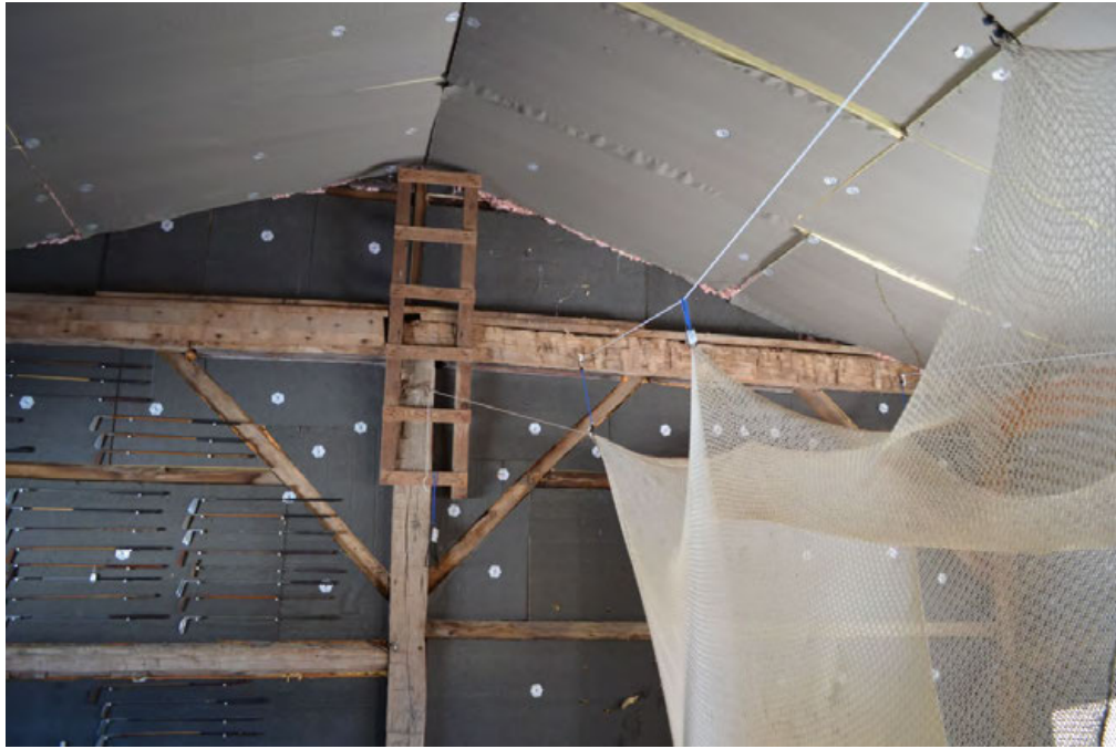
35. Interior of Barn I's south Addition II, showing framing details, camera facing east.
