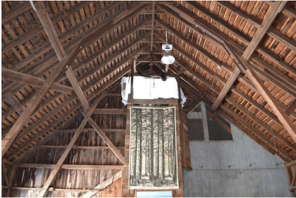
37. Interior of Barn I's west addition upper level, showing framing and roof details, camera facing east. Note hay chute at center and former exterior wall details at right.
