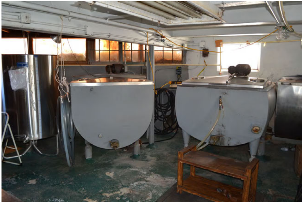
24. Interior of the Cider mill ground level, showing floor and framing details of eastern block, camera facing northeast. Note hard cider storage tank at far left, sweet cider tanks at center and right, steel girder at upper left.
