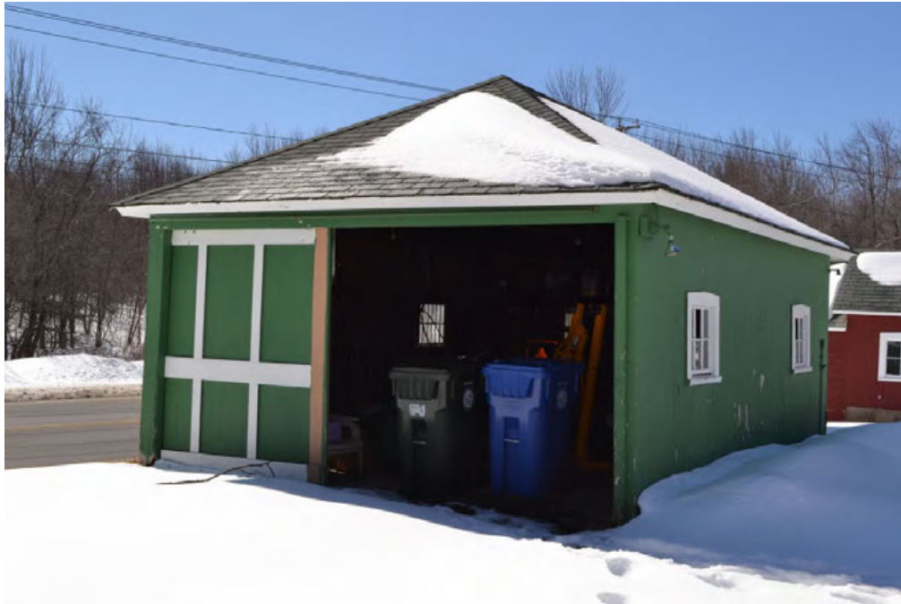
15. East and north eave-sides of Garage I, camera facing southwest. Note Milk house at rear right.
