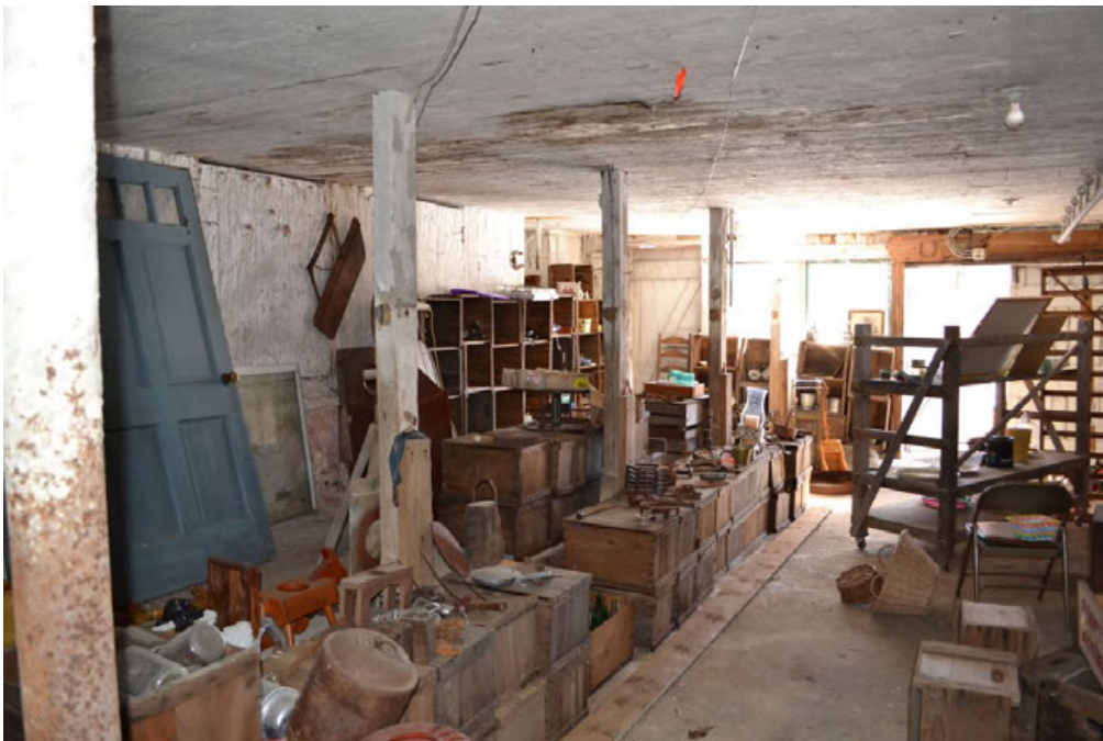
32. Interior of Barn I's south addition lower level, showing floor, post, wall, and ceiling details, camera facing south.
