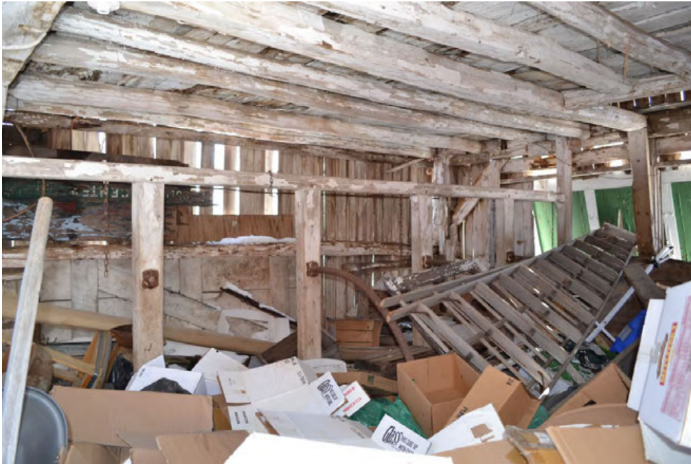
13. Interior of Barn II, showing framing and stanchion details, camera facing southeast.
