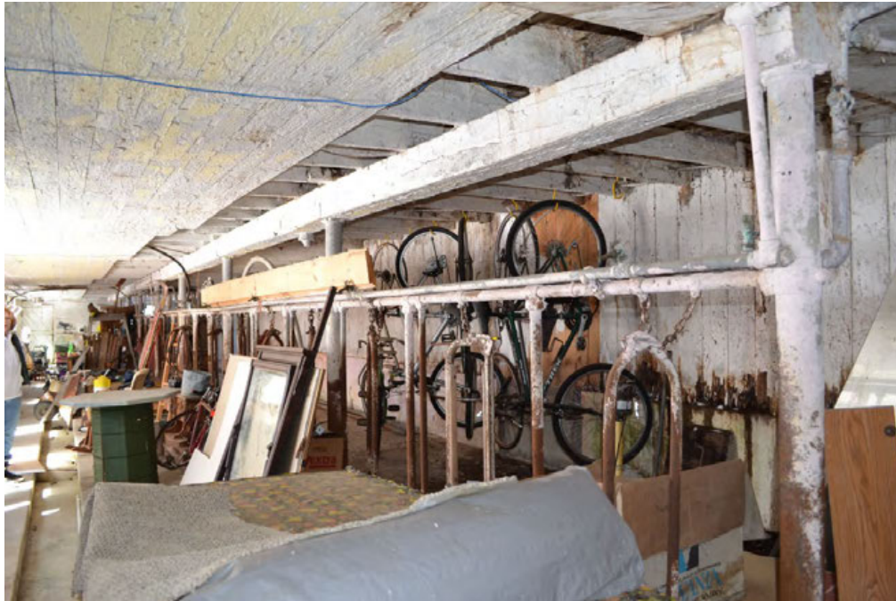
33. Interior of Barn I's central and western blocks lower level, showing floor, post, stanchion, girder, wall, and ceiling details, camera facing northwest.
