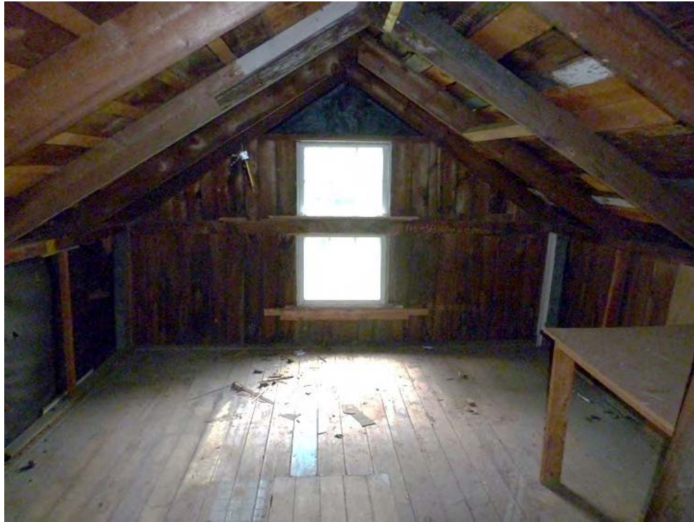
33. Interior view of the second floor east gable-end of Addition I, camera facing east.
