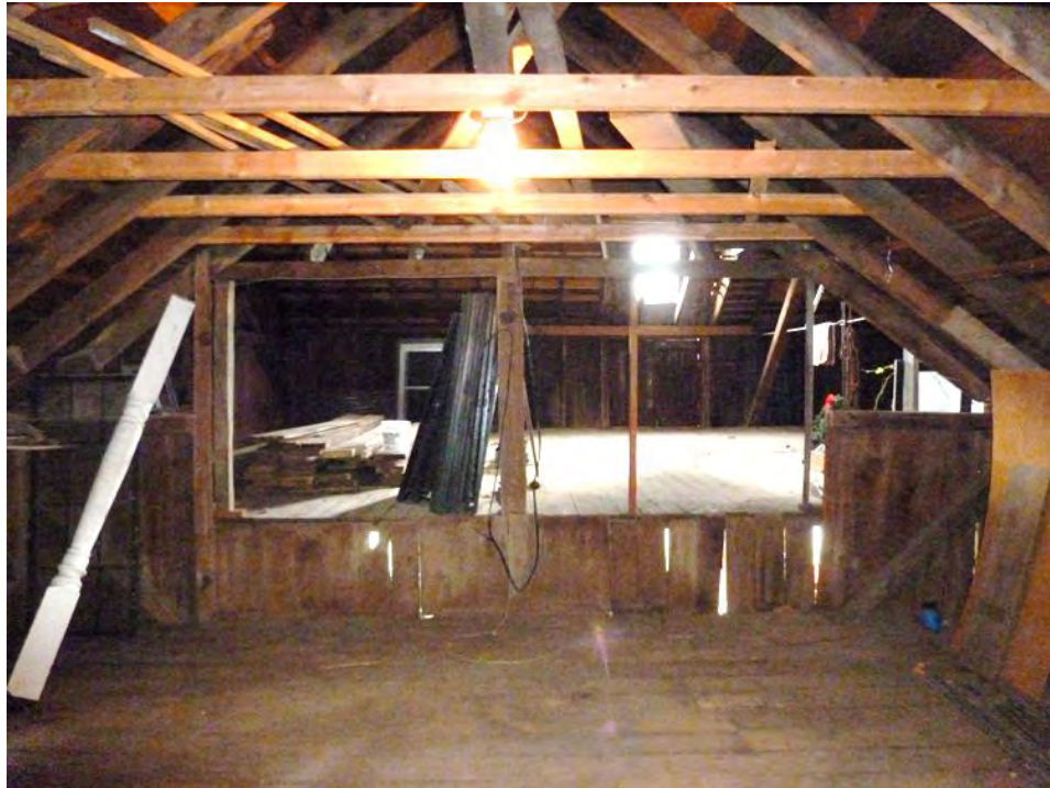
39. Interior view of the second floor of Addition III, note the rise in the floors and open bays that leads to the second floor of the main barn. Camera facing south.
