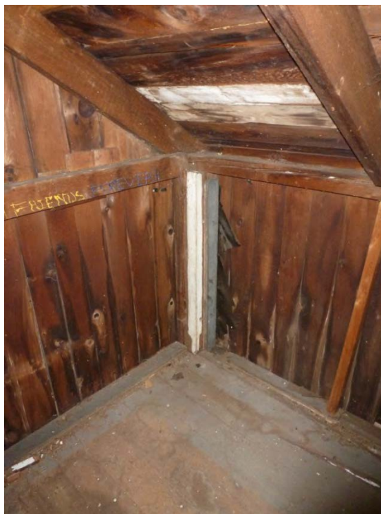
32. Interior view of the northeast corner of the second floor of Addition I, camera facing northeast.
