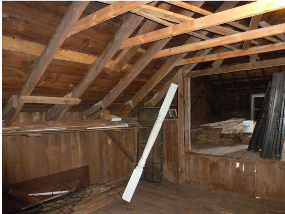
41. Interior view of the second floor southeast corner of Addition III, note the rafters from Addition II protruding through the wall, and collar ties helping to support the roof. Camera facing southeast.
