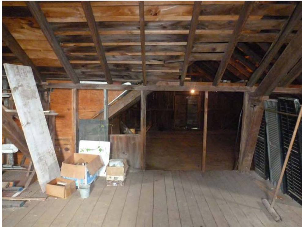
23. Interior view of the north side of the second floor of the barn, camera facing north.
