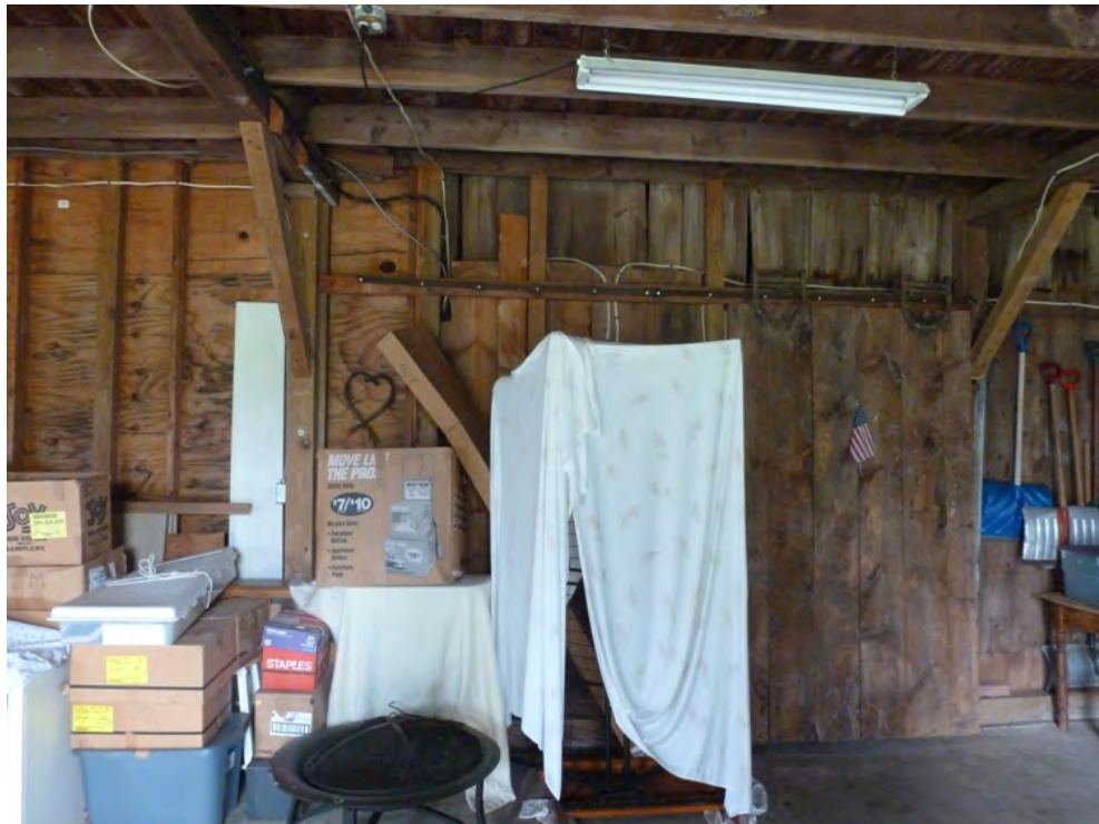
22. Interior view of the north wall of the barn, note the interior hung sliding door. Camera facing north.
