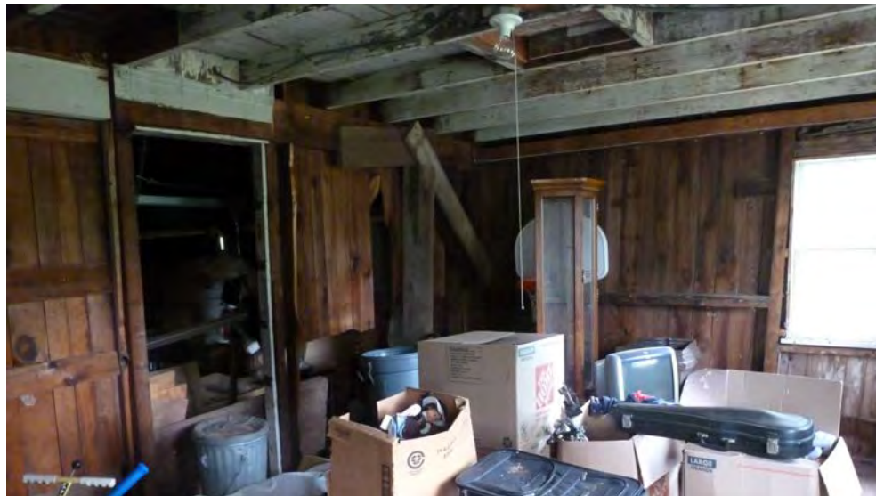
30. Interior view of Addition I, note the open doorway that leads into Addition II, camera facing northeast.
