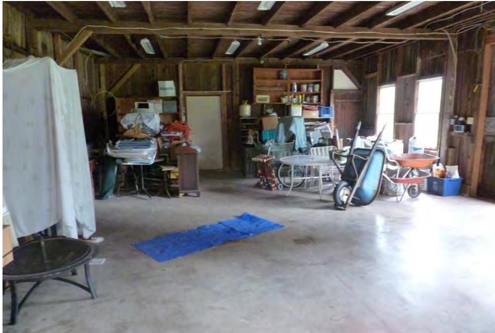
19. Interior view of the east half of the interior of the barn, camera facing east. Note the clear span without an interior post.
