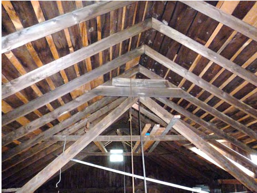
27. Interior view of the common rafters and roof deck of the barn, found on the second floor.
