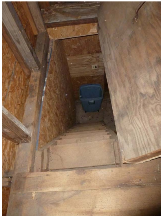
38. Interior view of the built in staircase in Addition III that leads to the second floor.
