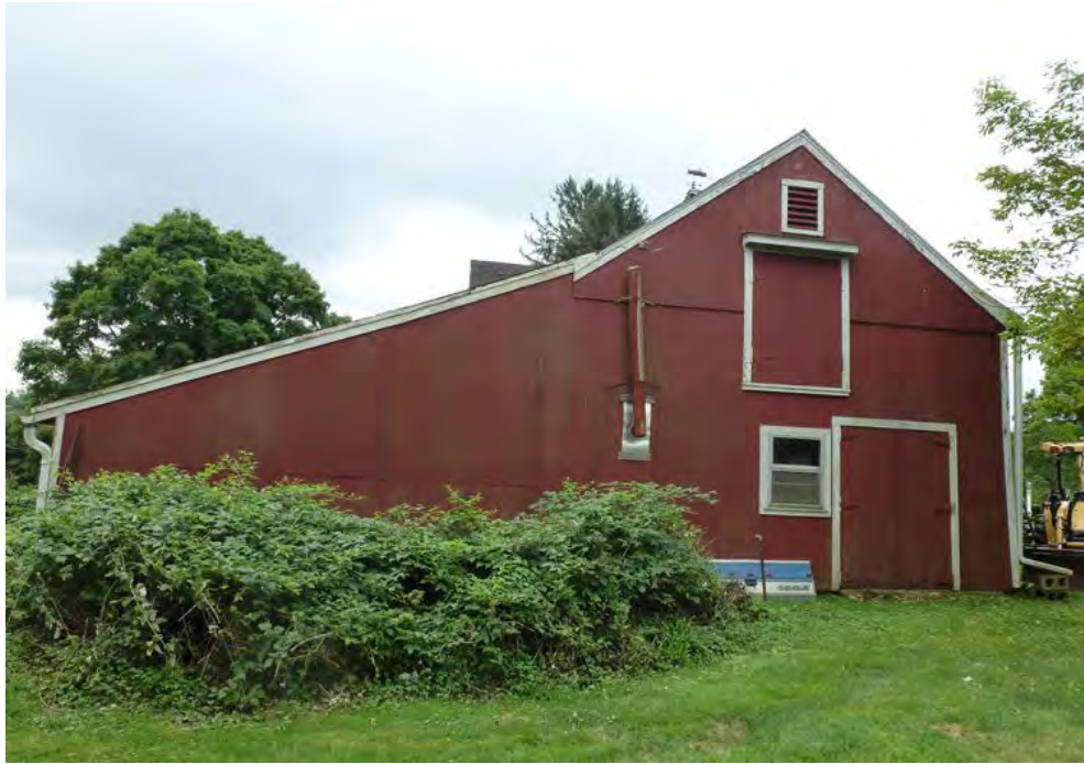
15. North side of Addition II and north gable-end of Addition III, camera facing south.
