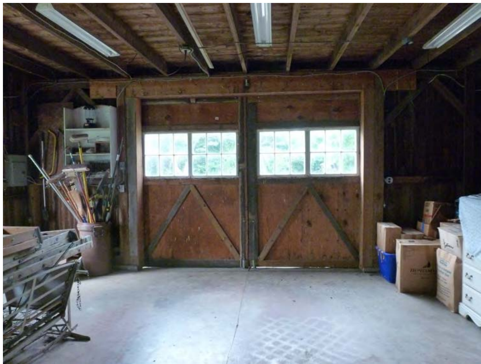
20. Interior view of the west half of the interior of the barn, camera facing west.
