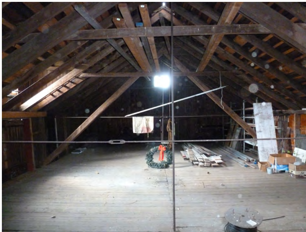
26. Interior view of the second floor west gable-end of the barn. Note the two sets of steel tension cables and the large diagonal truss frame helping to stabilize the barn and support the clear span below. Camera facing west.
