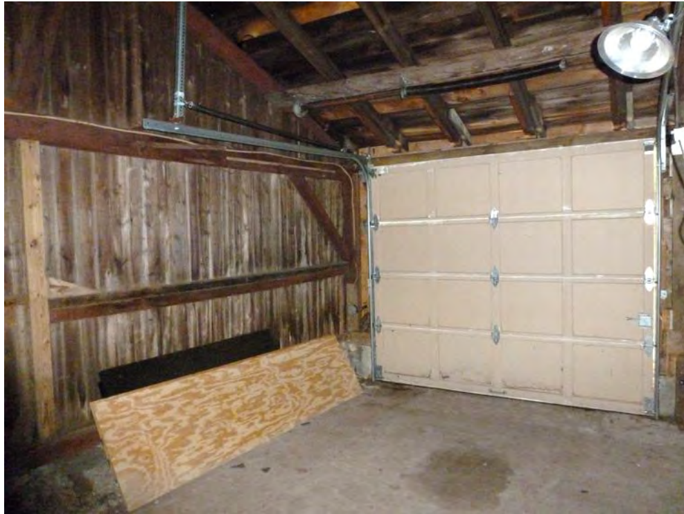
37. Interior view of the northeast corner of Addition II, camera facing northeast.
