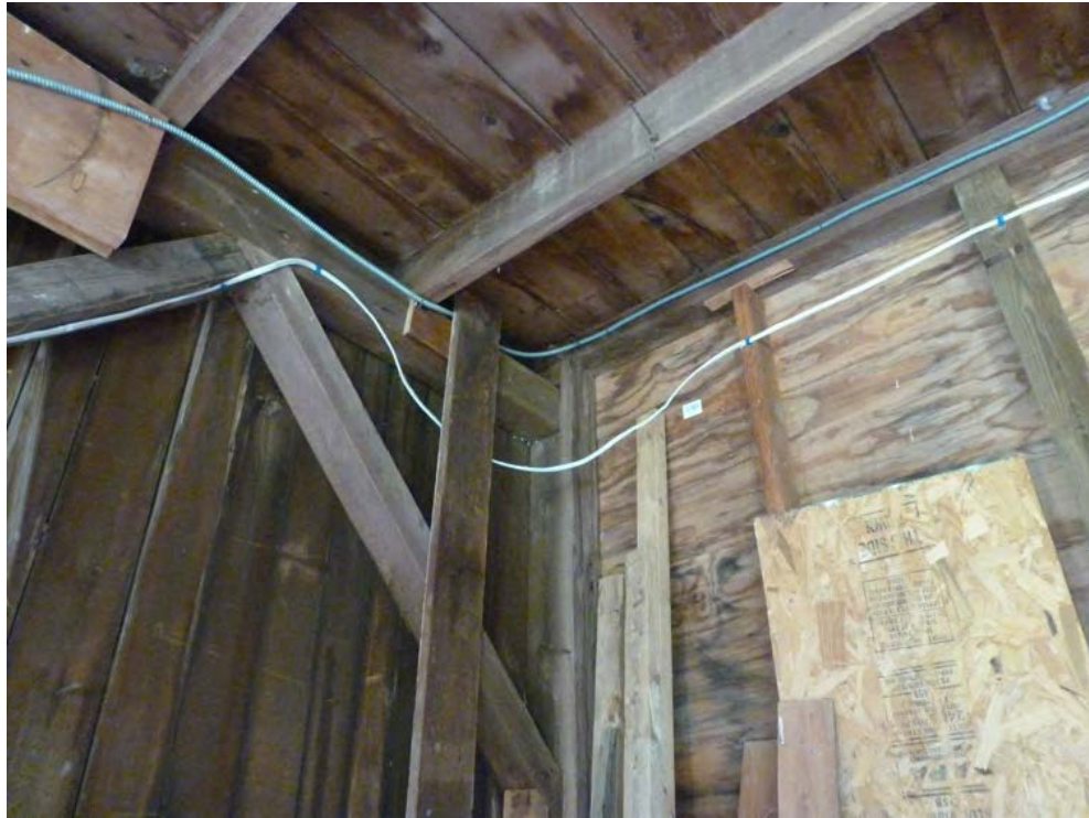
21. Interior view of the northwest corner of the barn, note the square rule post-and-beam framing, camera facing northwest.
