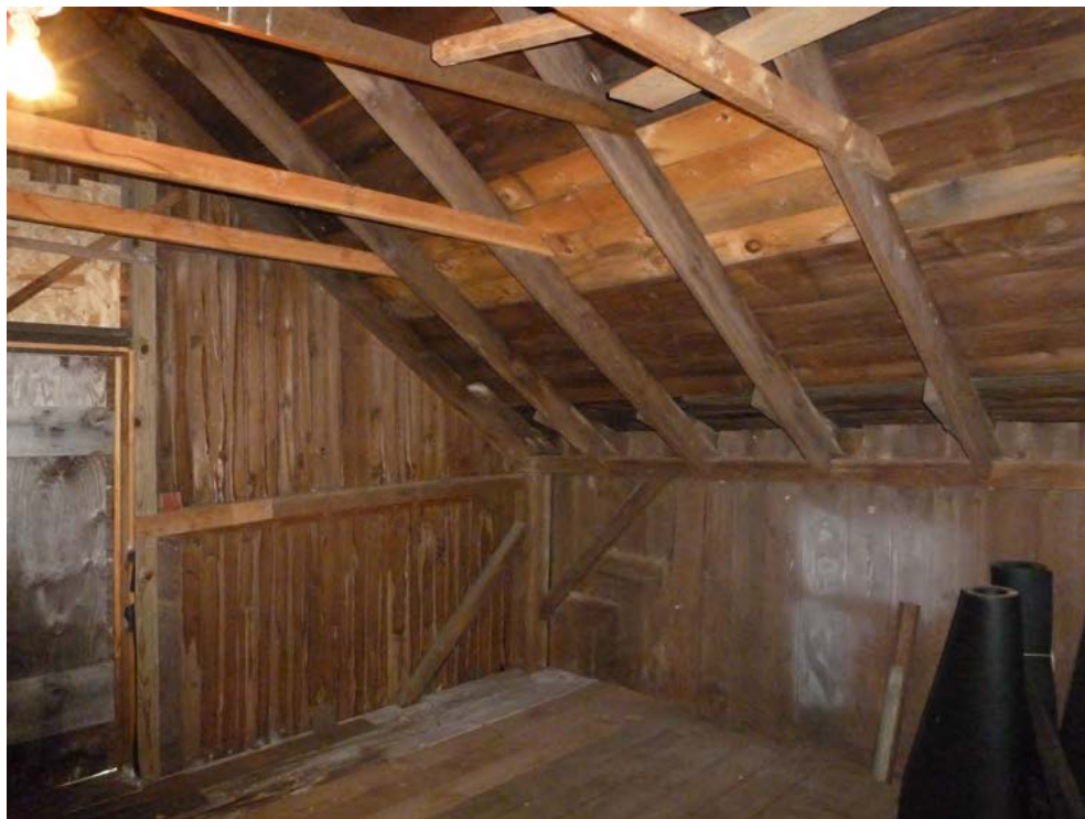
40. Interior view of the second floor northeast corner of Addition III, note the post-and-beam framing. Camera facing northeast.
