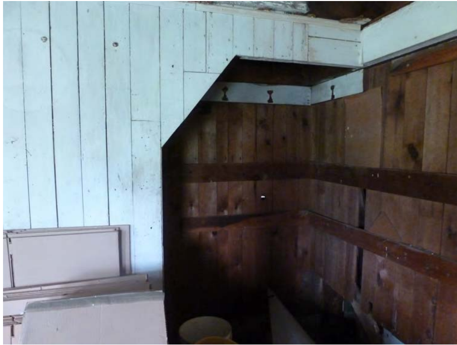
29. Interior view of the cubby behind the staircase in Addition I, camera facing northwest.
