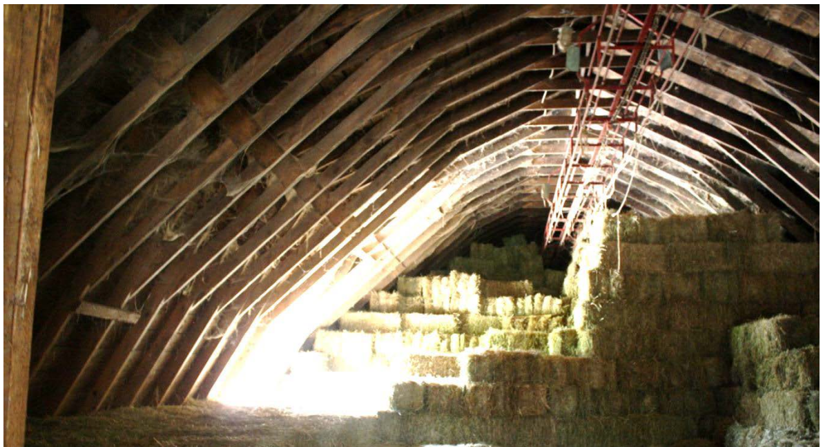
20. Interior view of Barn I Addition I loft level, camera facing south, showing gambrel roof construction and modern hay loading track.
