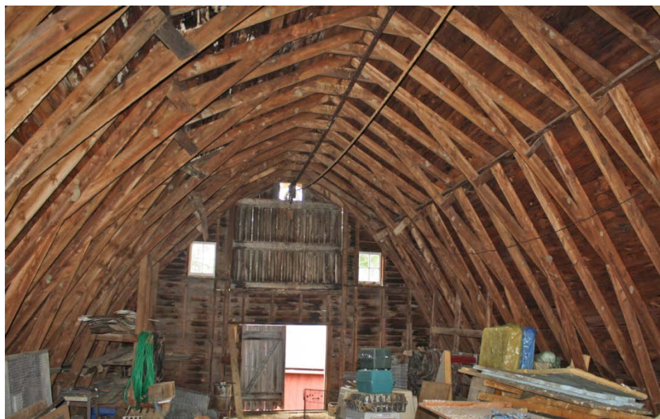
26. Interior view of Barn II loft level, camera facing south. Note the hay doors.
