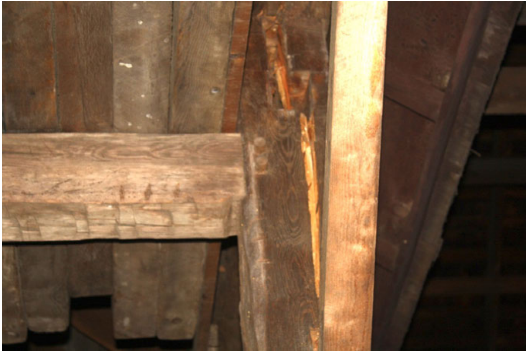
23. Detail of the interior of the Barn, hand hewn square rule construction, camera facing south.
