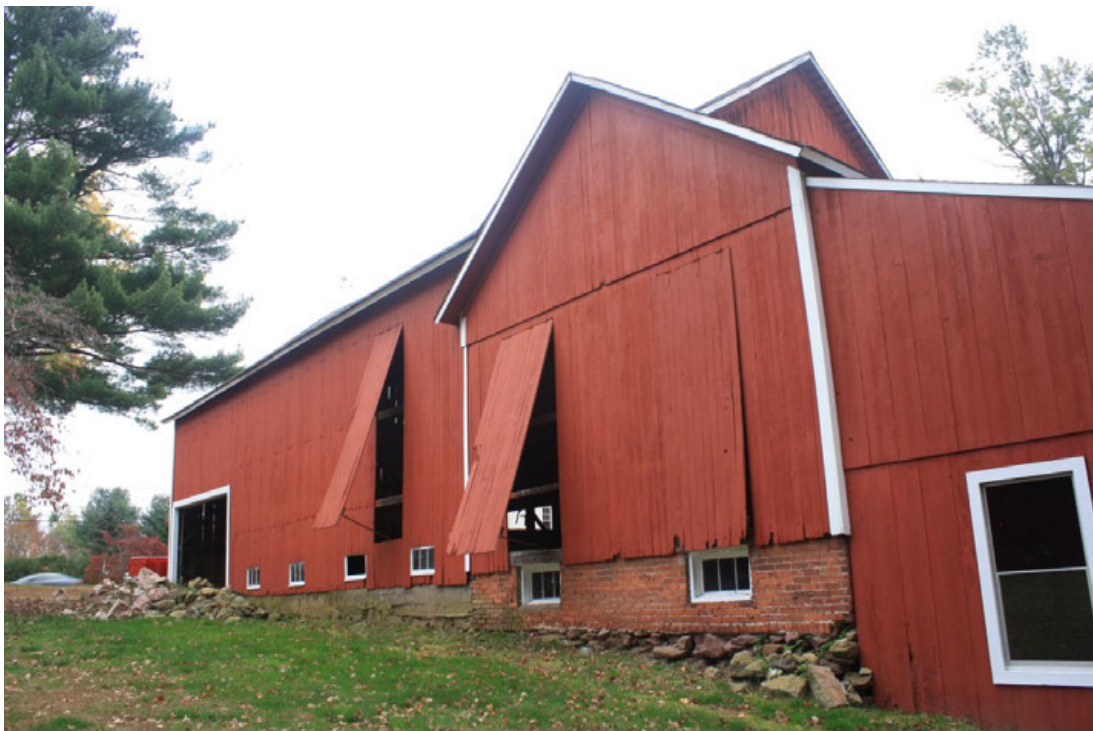
22. North eave-side of the barn, camera facing south. Note the top-hinged venting for tobacco curing.
