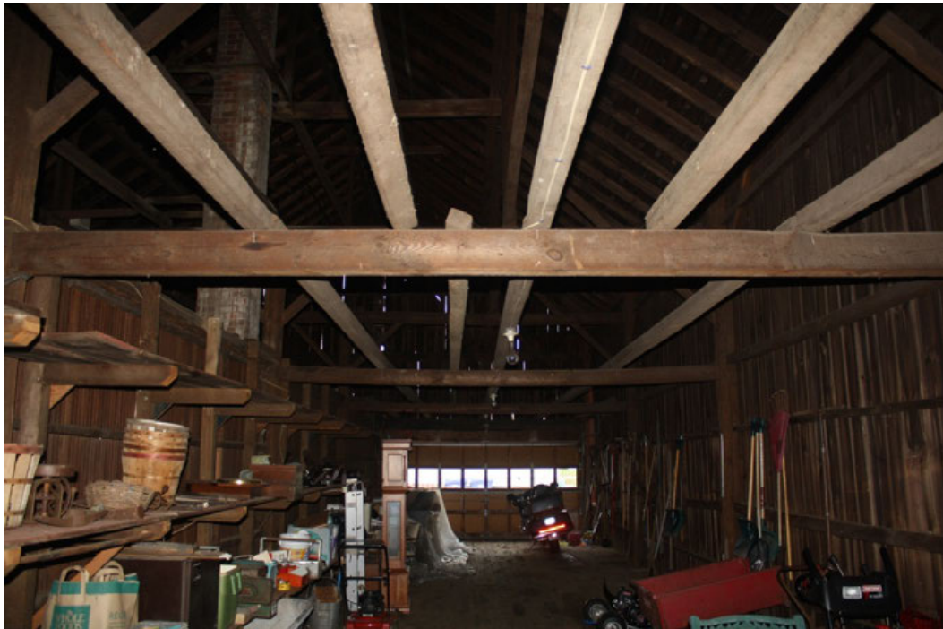
16. Detail of the interior of the Tobacco shed main level, south aisle, camera facing east. Note the rails for the tobacco still in place.
