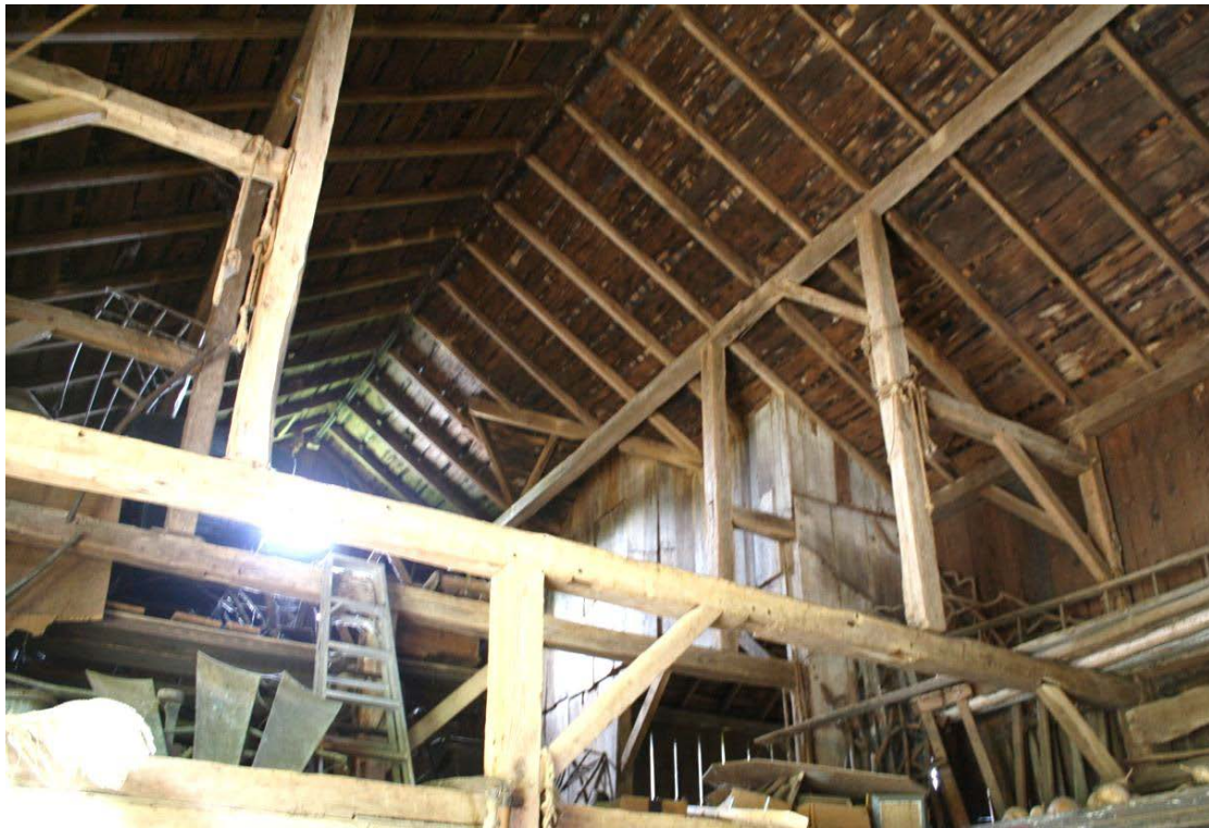
26. Interior view of Barn I, camera facing northeast from the threshing bay. Note the posts of the narrow bay set close together.
