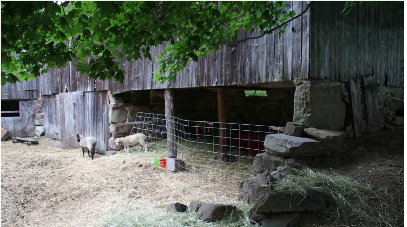
23. Southwest view of Barn II, camera facing northeast, showing basement foundation walls.
