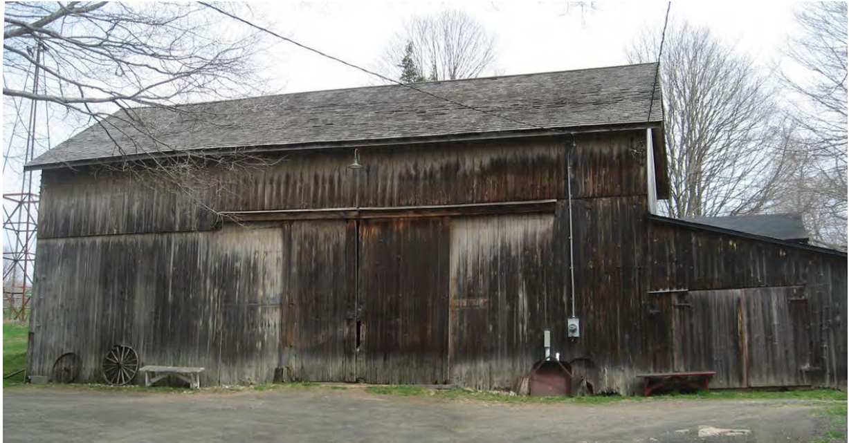
19. West view of Barn I (Erastus Dudley Barn), camera facing east. Note Windmill base at left rear.
