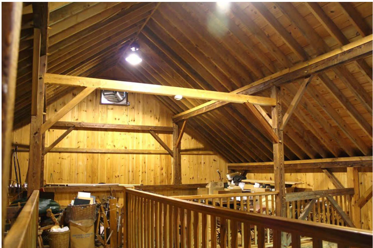
34. Interior view of Barn III loft level, camera facing east; in foreground is the "bridge" over the center bay.
