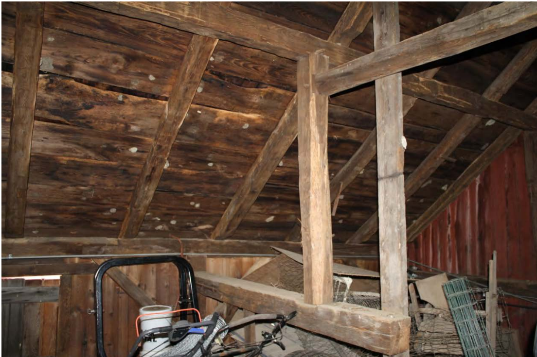
14. Interior view of Wagon Shed addition at south end of the Barn, loft level, camera facing northwest. Note the dropped tie-girt (center cut out for access), queen post, purlin plate, and hand-hewn rafters.
