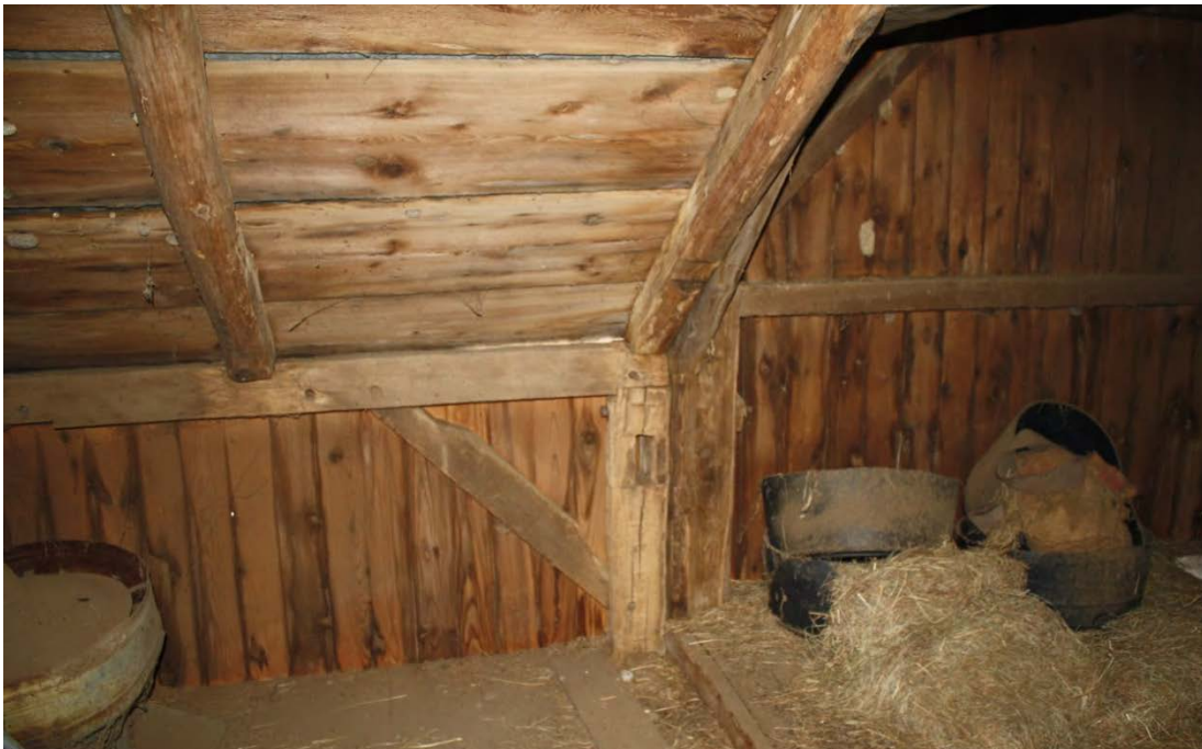
12. Interior view of Barn loft level, showing connection between central block and north addition, camera facing east. The double corner posts suggest that two complete barn structures were assembled abutting at the gable ends.
