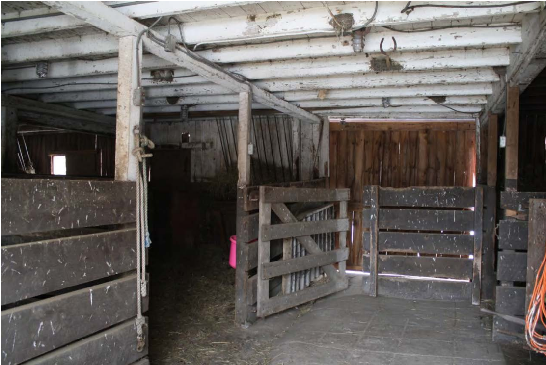
13. Interior view of Barn central block, ground level, camera facing east, showing horse stall configuration.
