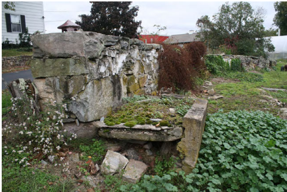
9. Southwest view of foundation wall of former greenhouse, camera facing northeast. Heating pipes ran underground along the north wall.
