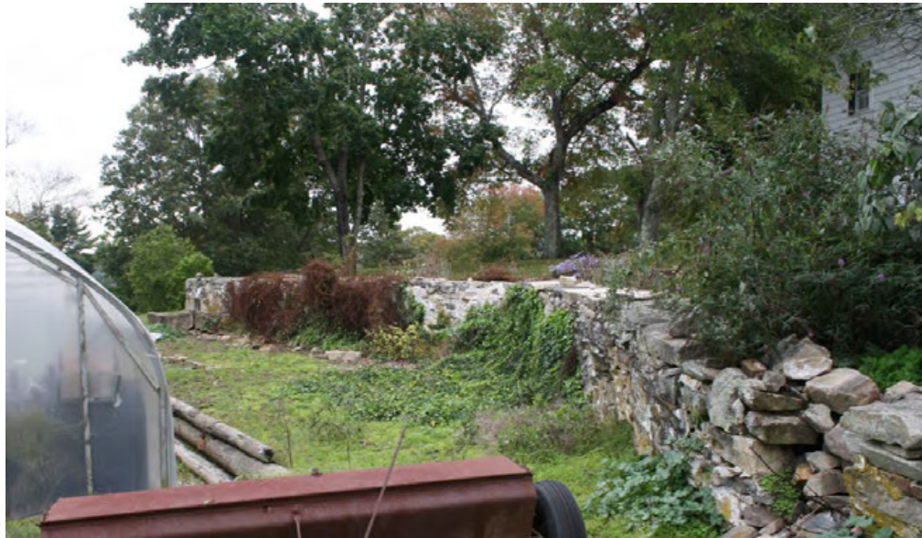
8. Southeast view of foundation wall of former greenhouse, camera facing northwest; Farmhouse at right rear.
