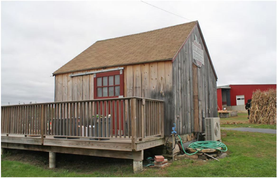
12. Southwest view of Barn I, camera facing northeast; Coop I / Apple storage is at right rear.
