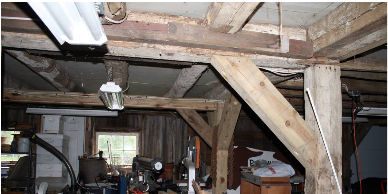
15. Interior of basement below threshing bay, camera facing south. Note change of joist direction in adjacent bay to right (west).
