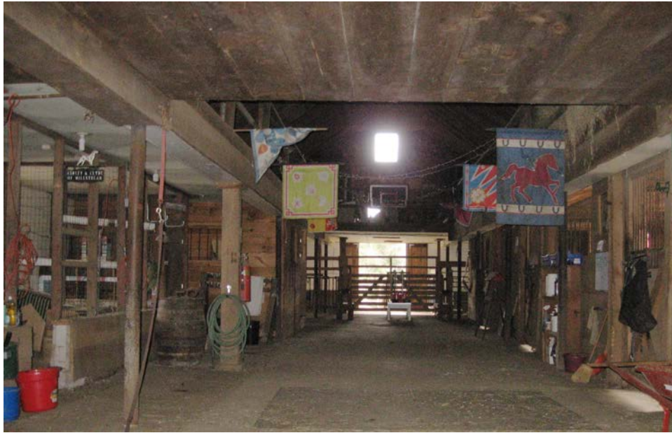
15. Interior view of Barn ground level, showing concrete floor, open ceiling and horse stalls, camera facing east. Note goat pens at rear.
