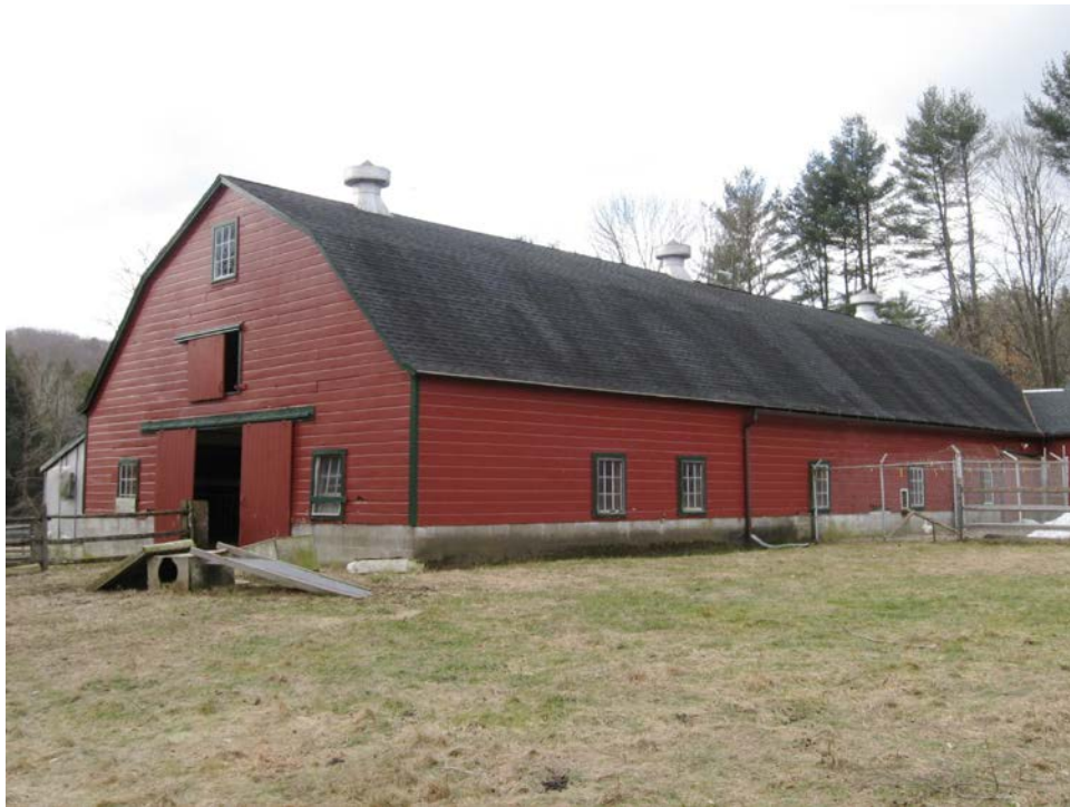
14. Northeast view of Barn, camera facing southwest. Note sliding hay door on gable end and ridge-line ventilators.
