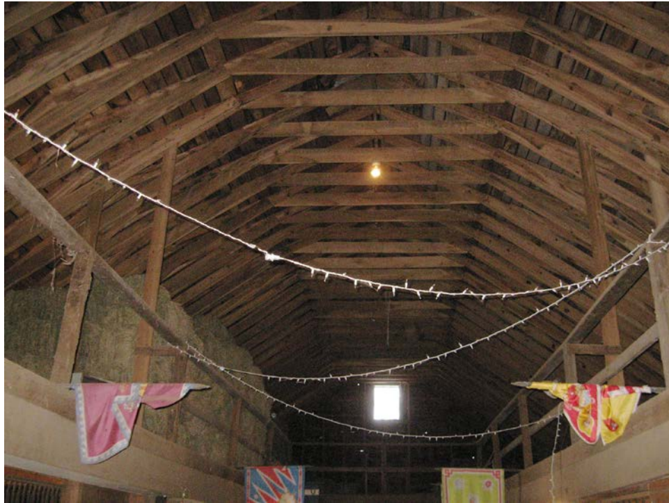
17. Interior view of Barn loft level, showing framing details, camera facing west.
