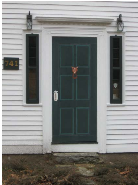
8. Farmhouse entry details, camera facing south. Note sidelights, molded surround, and denticulated entablature.
