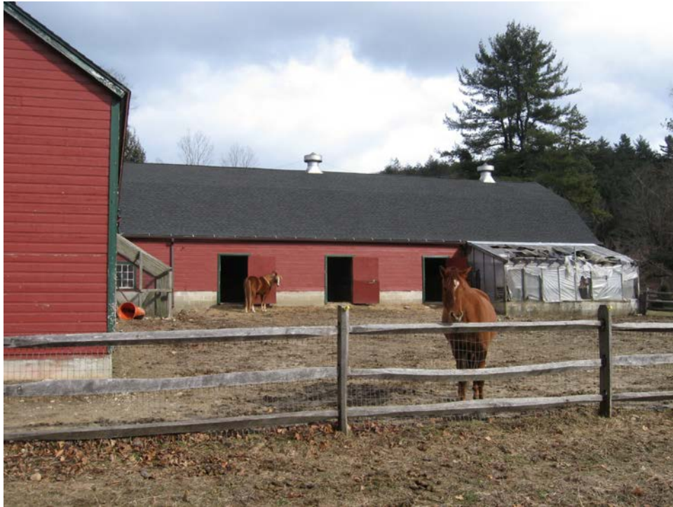
13. South eave-side of Barn and south corner of Addition II, camera facing northeast.
