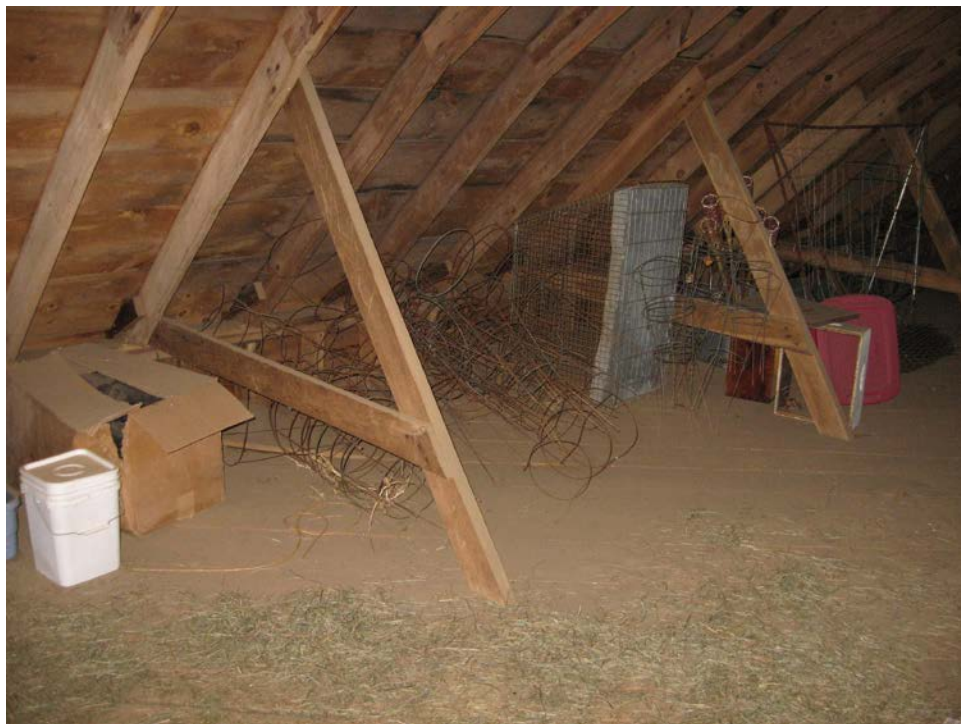
18. Interior view of Barn loft level, showing framing details, camera facing northeast. Note diagonal bracing, cross ties, and low knee wall.
