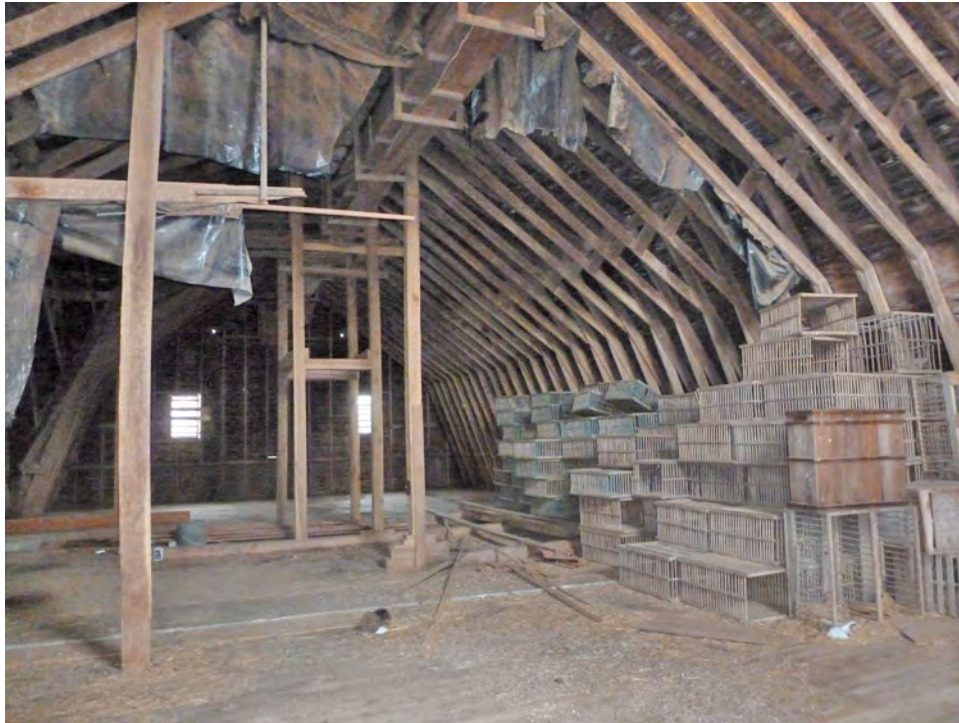
23. Interior view of the west gable-end of the north section of the loft of Barn I. Camera facing west.
