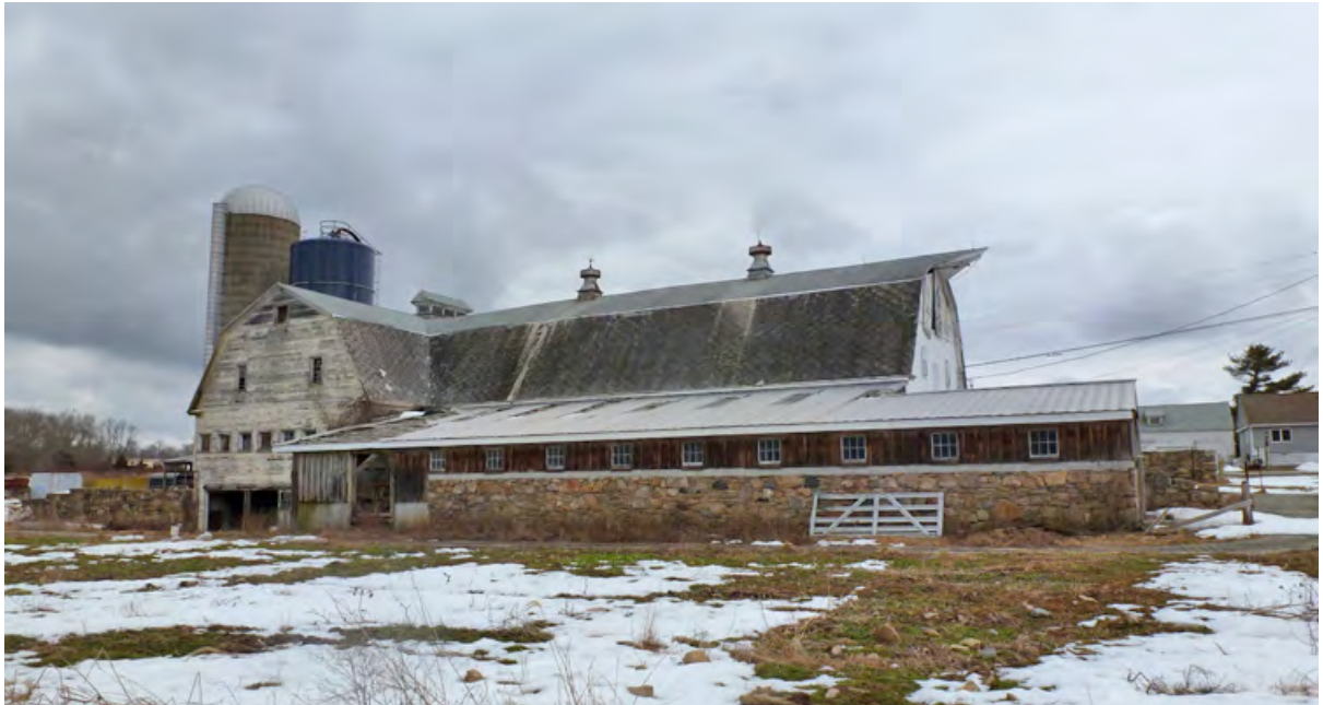
19. West gable-end of the north section and west eave-side of the south section of Barn I. Camera facing east.
