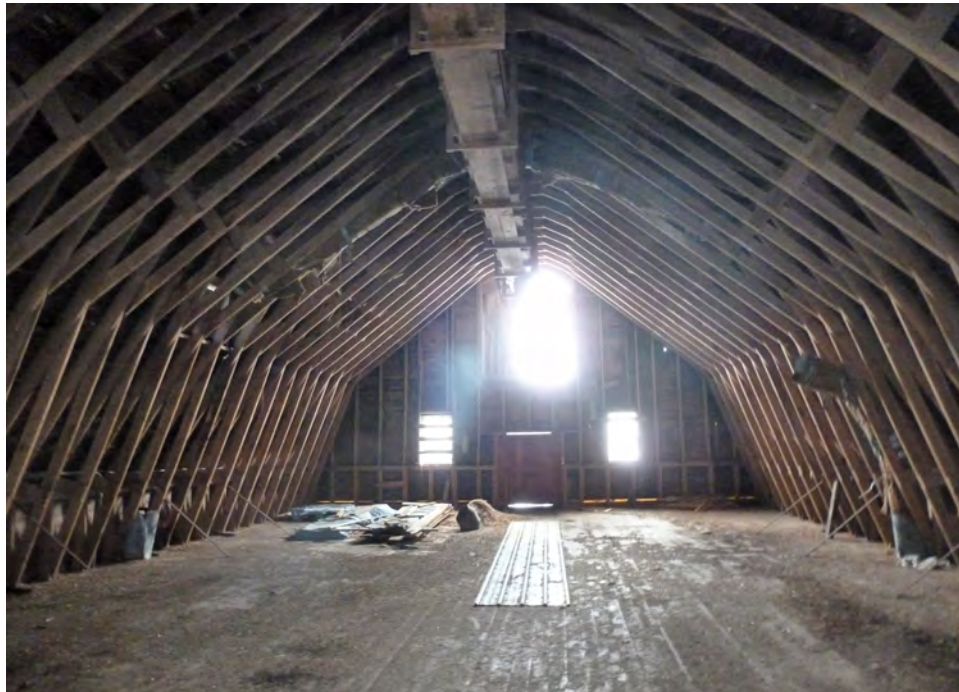
22. Interior view of the south gable-end of the south section of the loft of Barn I. Camera facing south. Note the typical scissor truss framing using sawn dimension lumber.
