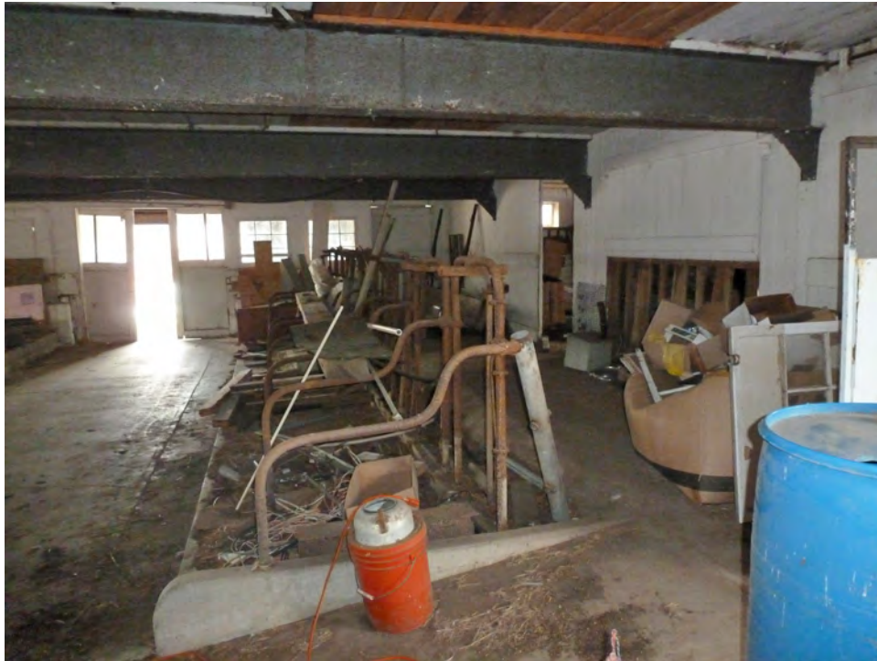
21. Interior view of the cow stanchions in the first story of the north section of Barn I. Camera facing north. Note the use of steel beams to create a clear-span space.
