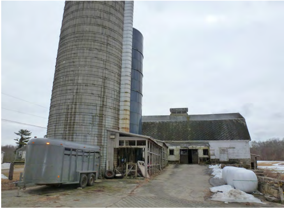
15. North eave-side of the north section of Barn I and Silos. Camera facing south.
