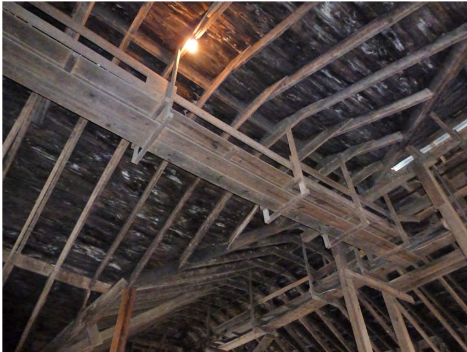
24. Interior view of the hay carrier track in the loft of Barn I. Note the ridge-board where the rafters meet. Camera facing north.
