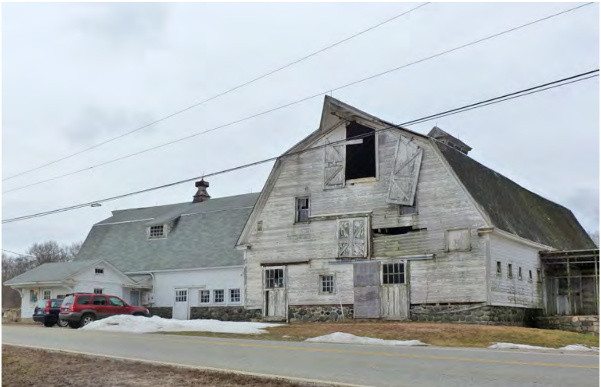
14. East eave-side of the south section, and east gable-end and north eave-side of the north section of Barn I. Camera facing southwest.
