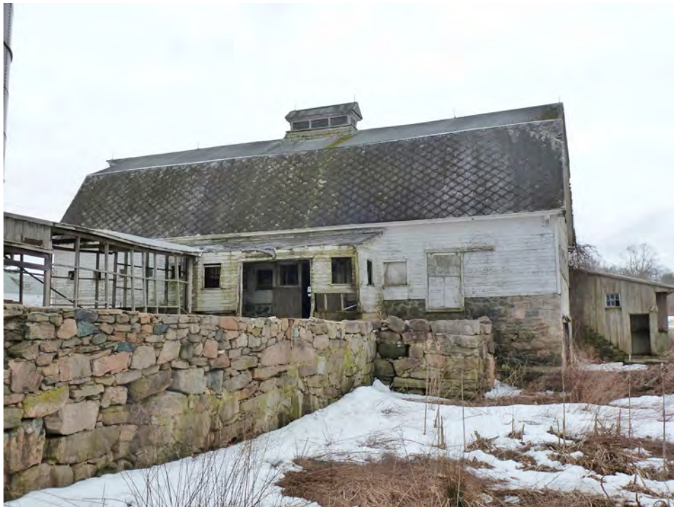
16. Close up of the north eave-side of the north section of Barn I. Camera facing south.
