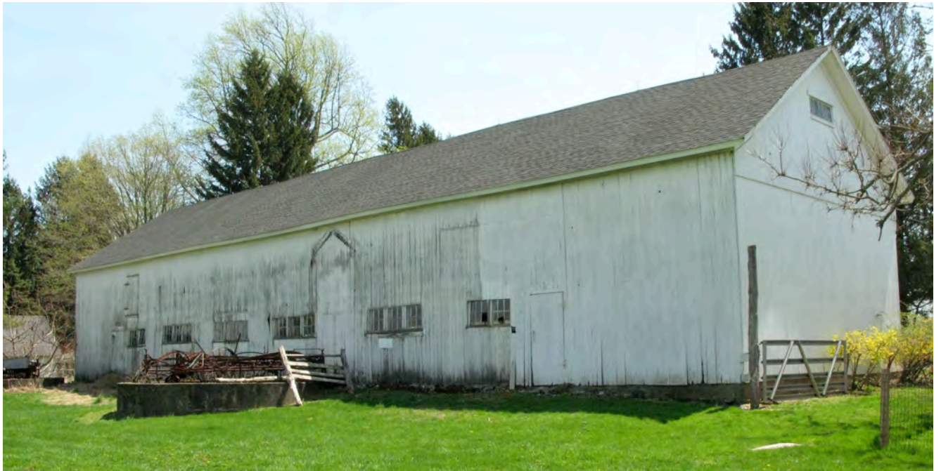
8. Northwest view of Barn, camera facing southeast. Note silo foundations (Gould photo).
