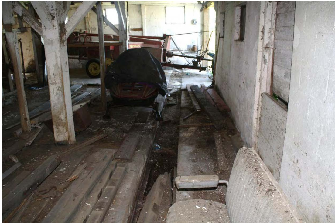
22. Detail of interior, manure trough in basement of Barn I, camera facing west. Note whitewash finishes, indicating use as a dairy stable.
