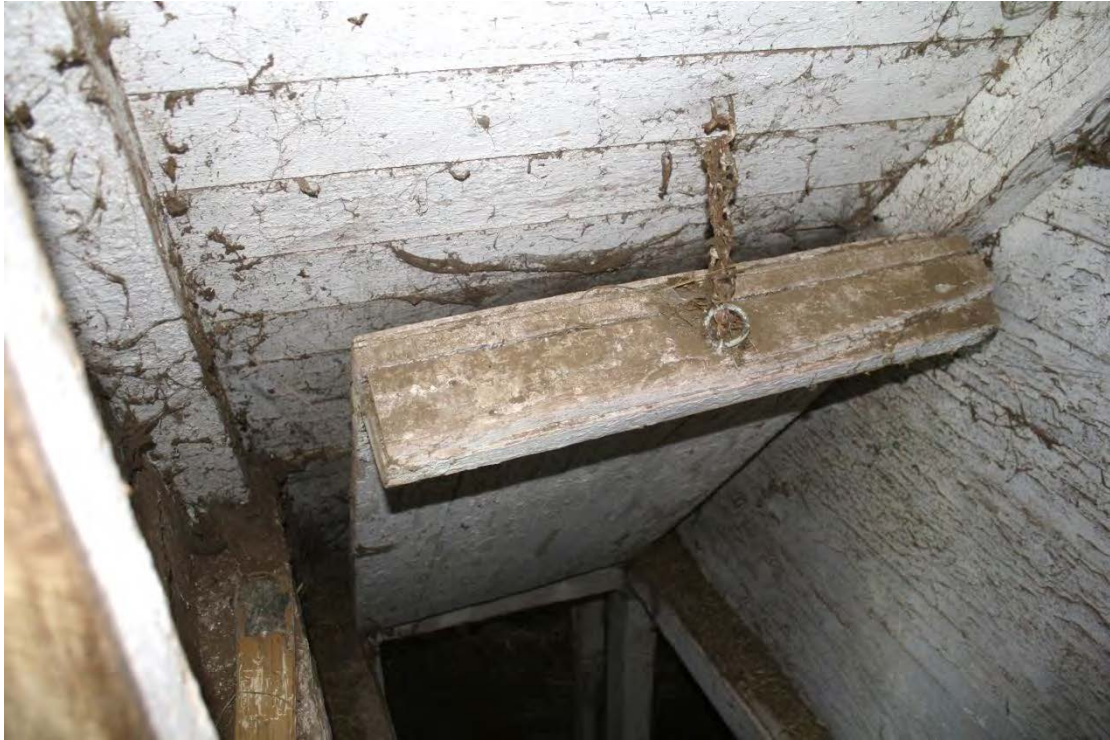
21. Detail of interior, hatch from main level to basement of Barn I, camera facing south.
