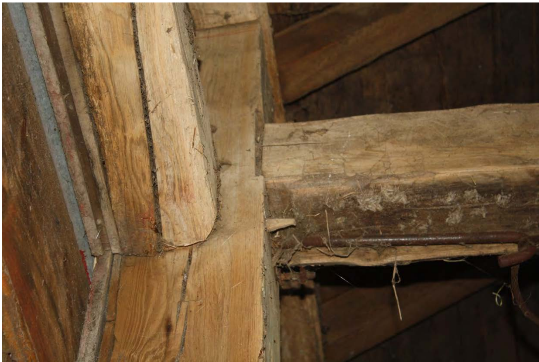
18. Detail of interior, square rule construction of Barn I, camera facing east.
