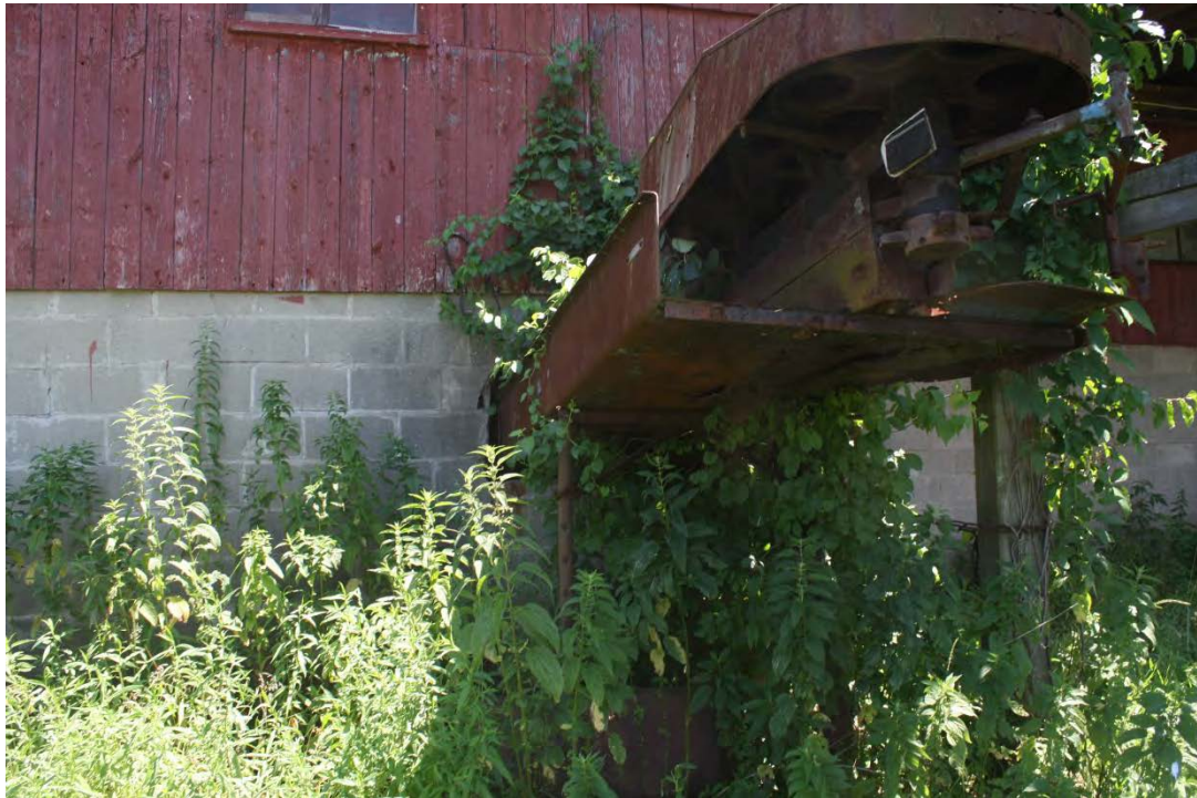
15. Detail of exterior, manure cleaner emerging through concrete block masonry foundation of Addition III, camera facing east.
