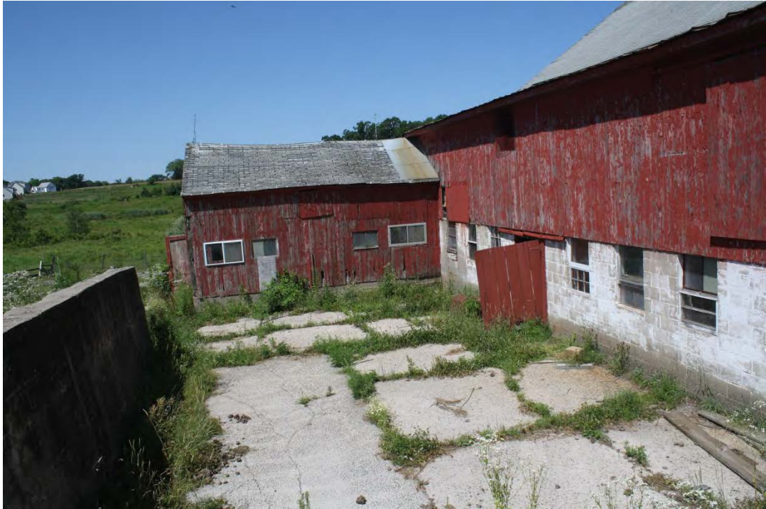
11. East eave-side of Addition II, south side of Addition I and retaining wall to the left, camera facing west.
