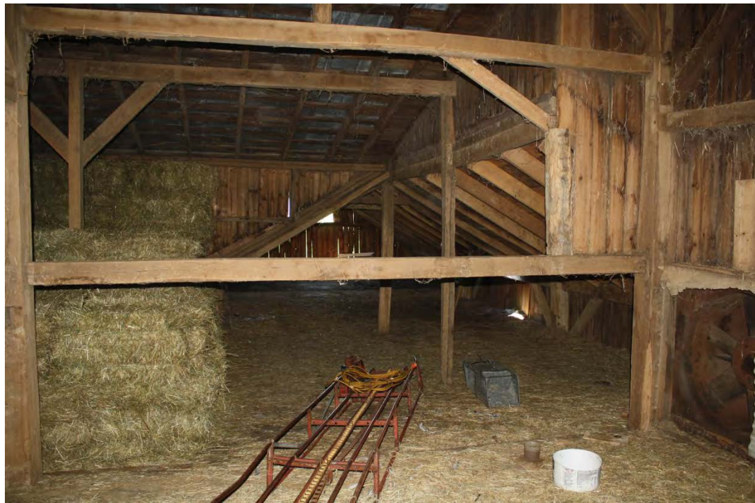
20. Detail of interior, transition space from Barn I to Addition II, camera facing south.
