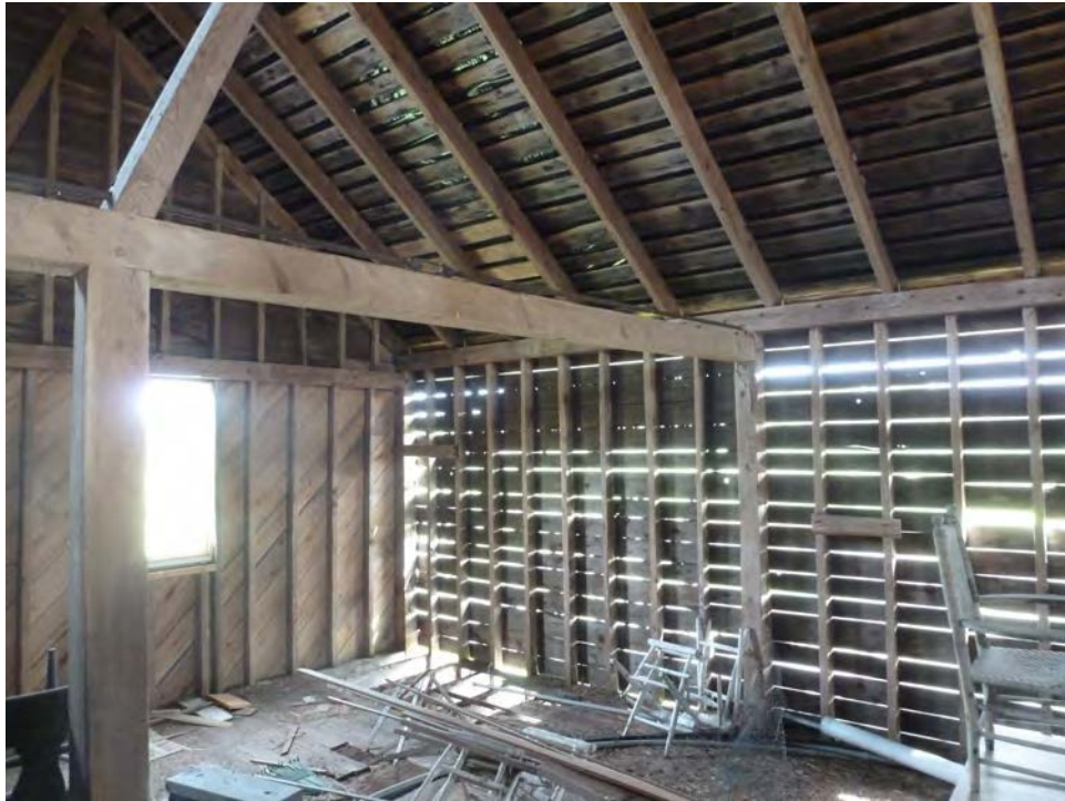
15. Interior view of the northeast corner of the Barn. Note the hybrid frame of heavy timber post and beam frame and lighter wood studs typically found in balloon frames. Camera facing northeast.
