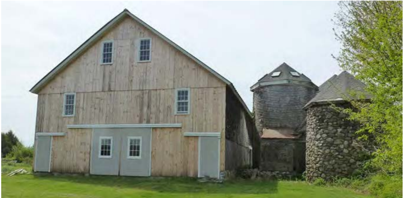
11. West eave-side and north gable-end of the Barn with Silos I and III (at right). Camera facing southeast.
