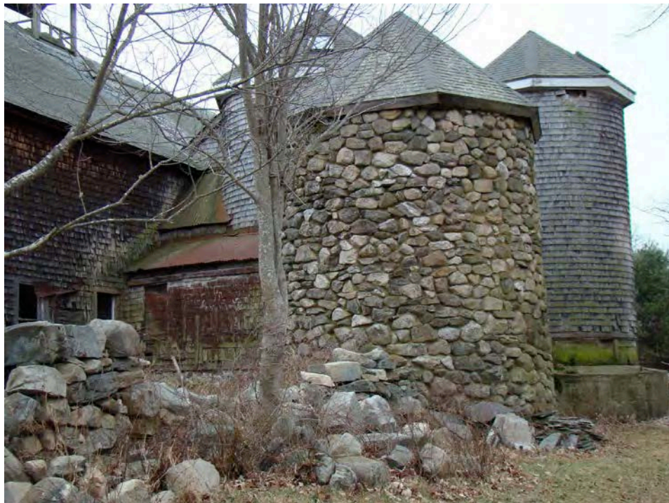
22. Southeast view of the Barn and Silos, prior to restoration work, showing connecting sheds between Silo I and Barn.
