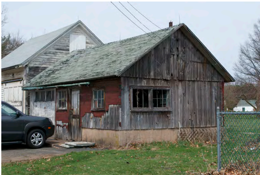
15. West eave-side and south gable-end of Bottling shed, camera facing northeast. Note Garage at left.
