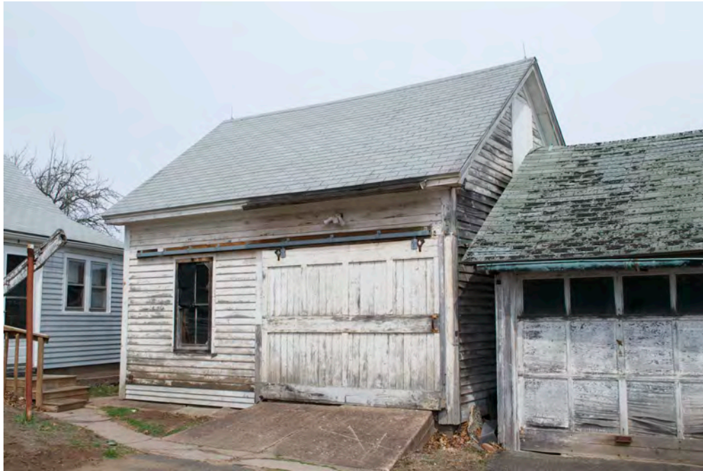
14. West eave-side and south gable-end of Garage, camera facing northeast. Note Farmhouse I rear porch at left, Bottling shed at right.
