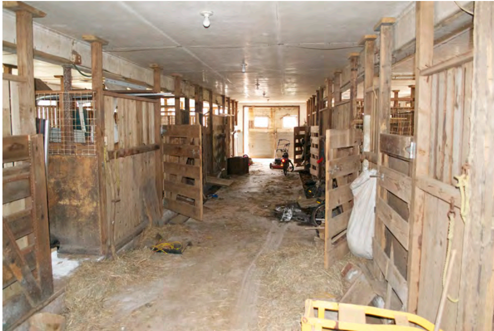
30. Interior of Barn rear ell, showing dairy central aisle details, camera facing south. Note horse stalls flanking aisle, finished ceiling.
