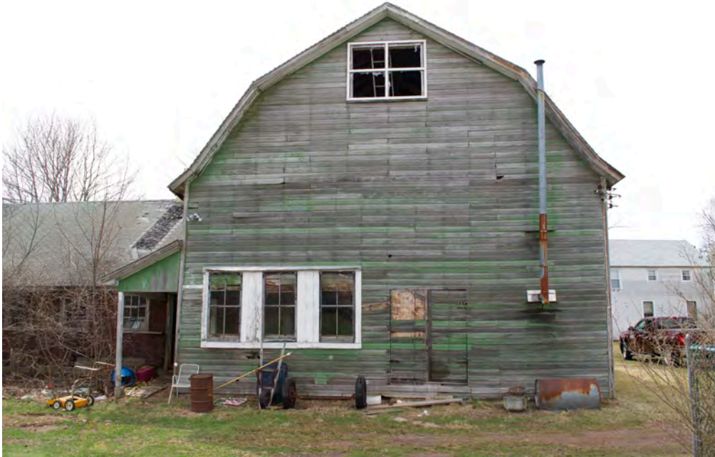
22. East gable-end of Barn, camera facing west. Note entry porch at left.
