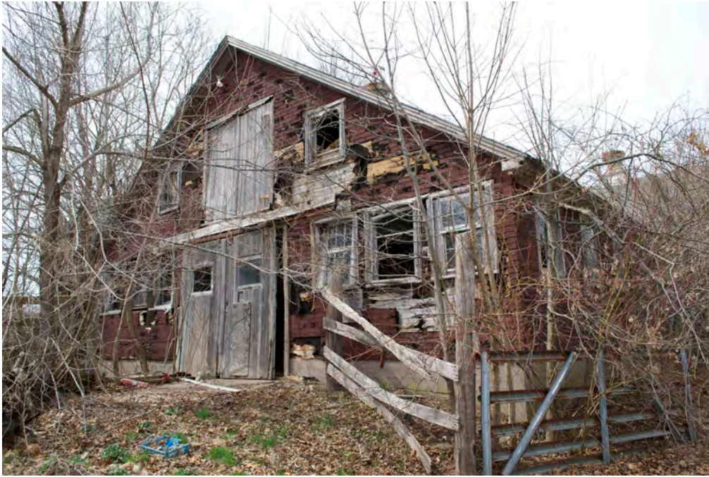
24. South gable-end of Barn, camera facing northwest. Note earthen ramp leading to centered entry doors, hay doors above.
