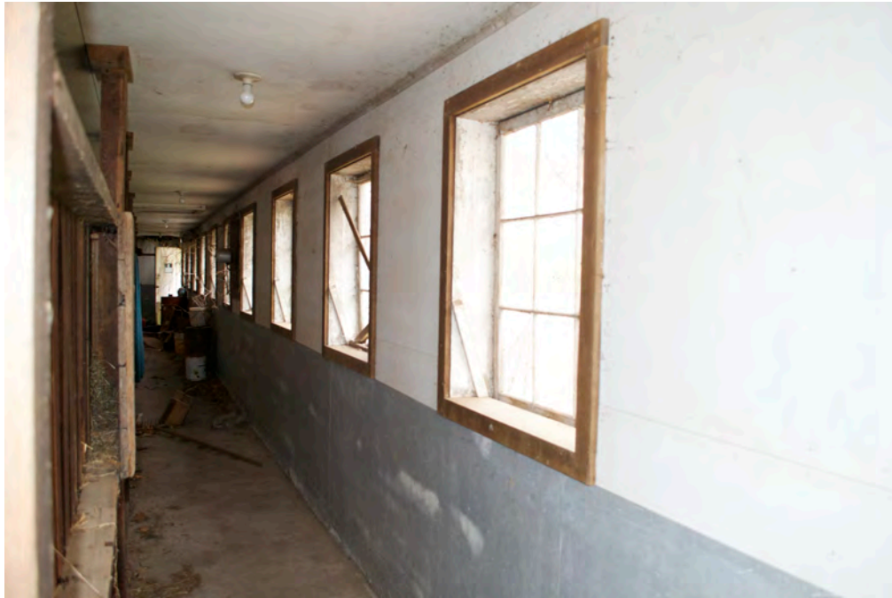
32. Interior of Barn rear ell, showing east eave-side window details, camera facing northeast. Note finished walls, nine-pane hopper windows.
