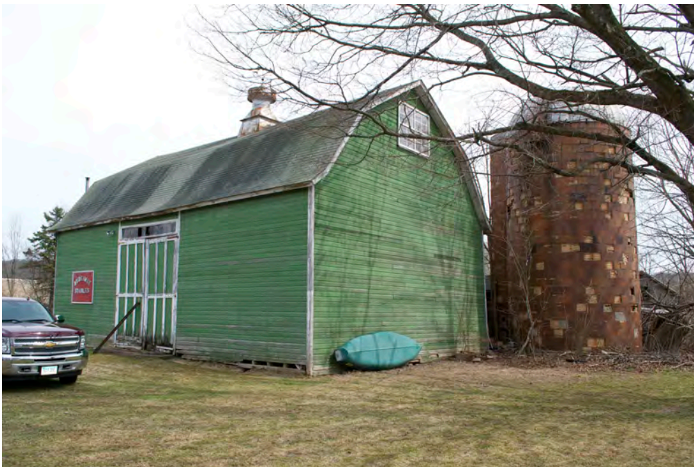
25. North eave-side and west gable-end of Barn, camera facing southeast. Note Silo at right.
