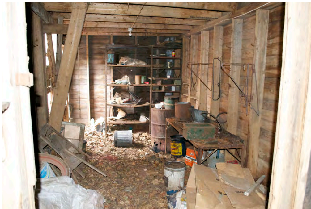
29. Interior of Barn main block, showing storage area at southwest corner of main block, camera facing west.
