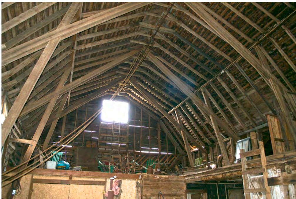
27. Interior of Barn main block, showing interior details, camera facing east. Note scissor trusses.
