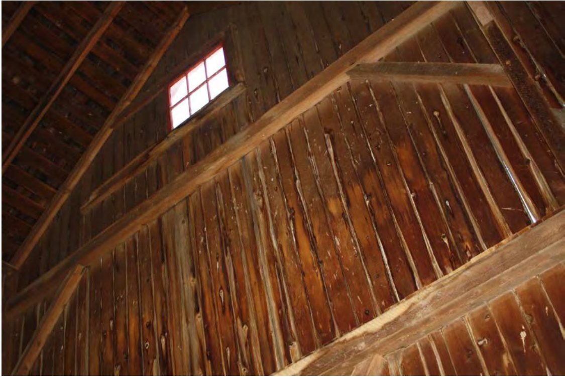
15. Detail of interior main level of Barn I, showing gable-end with dropped girt.
