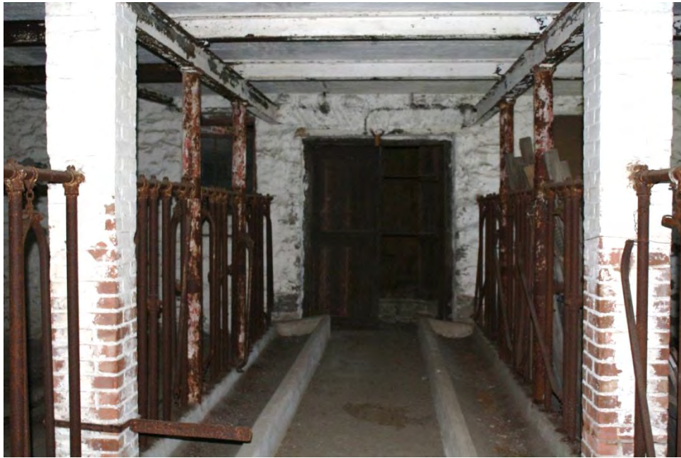
31. Detail of the interior of the first (basement) level of Barn III, camera facing north. Note cow stanchions on both sides of the center aisle.
