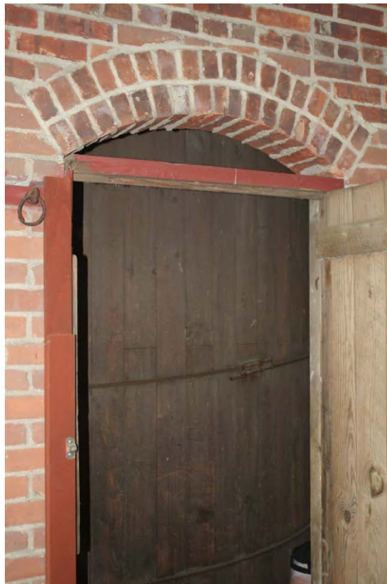
32. Doorway on the east side of Addition III that leads to the wooden silo, camera facing west.
