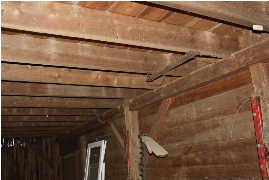
16. Detail of the interior of Barn II, band saw kerf marks on the ceiling boards, camera facing north.
