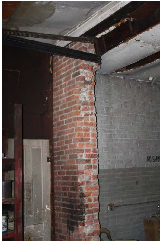
27. Detail of the damaged interior bays of the third and top level of Barn III, with the doors removed, camera facing east.
