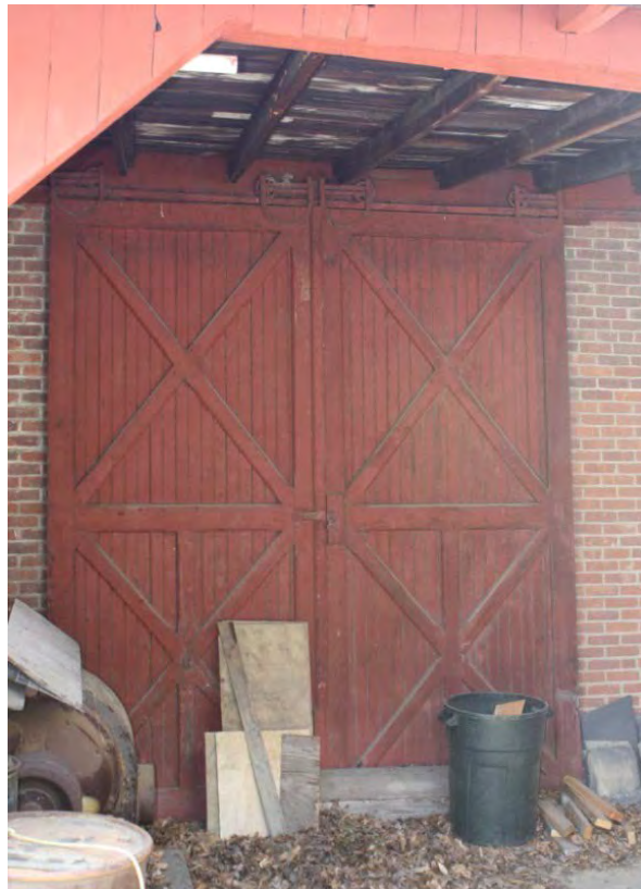
20. Detail of the original doors on the east eave-side third level of Barn III, still extant under the roof of Addition II, camera facing west.
