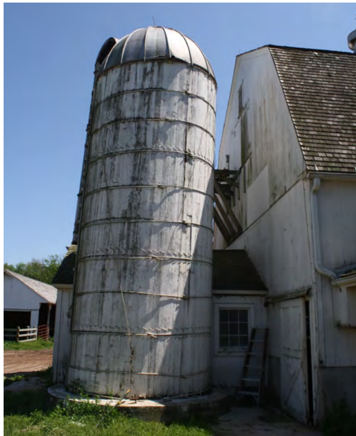
6. West side of silo, camera facing east. Note cleats holding the vertical boards of the silo together.
