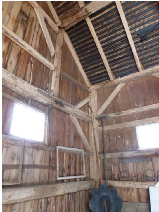
16. Interior view of the northwest corner of the Barn and the post-and-beam frame. Note the dropped tie girt. Camera facing northwest.
