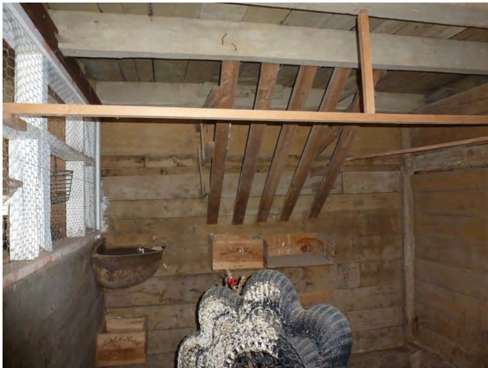
18. Interior view of the extant manger in the east gable-end of the Barn. Camera facing west.
