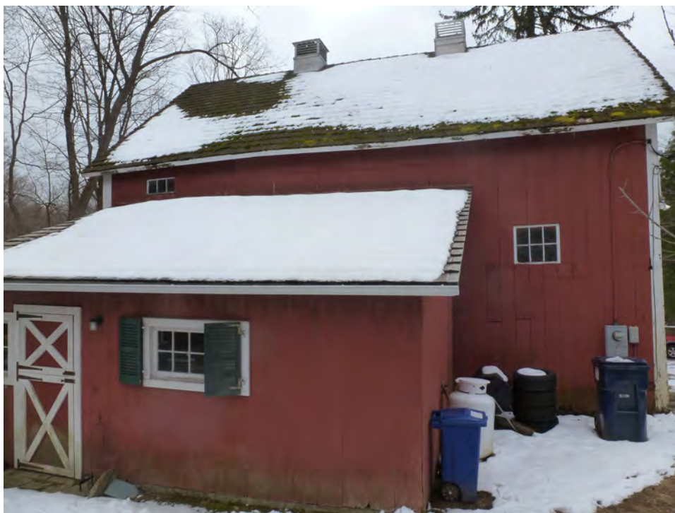
12. North eave-side of the Barn and north eave-side of shed-roof addition. Camera facing south.
