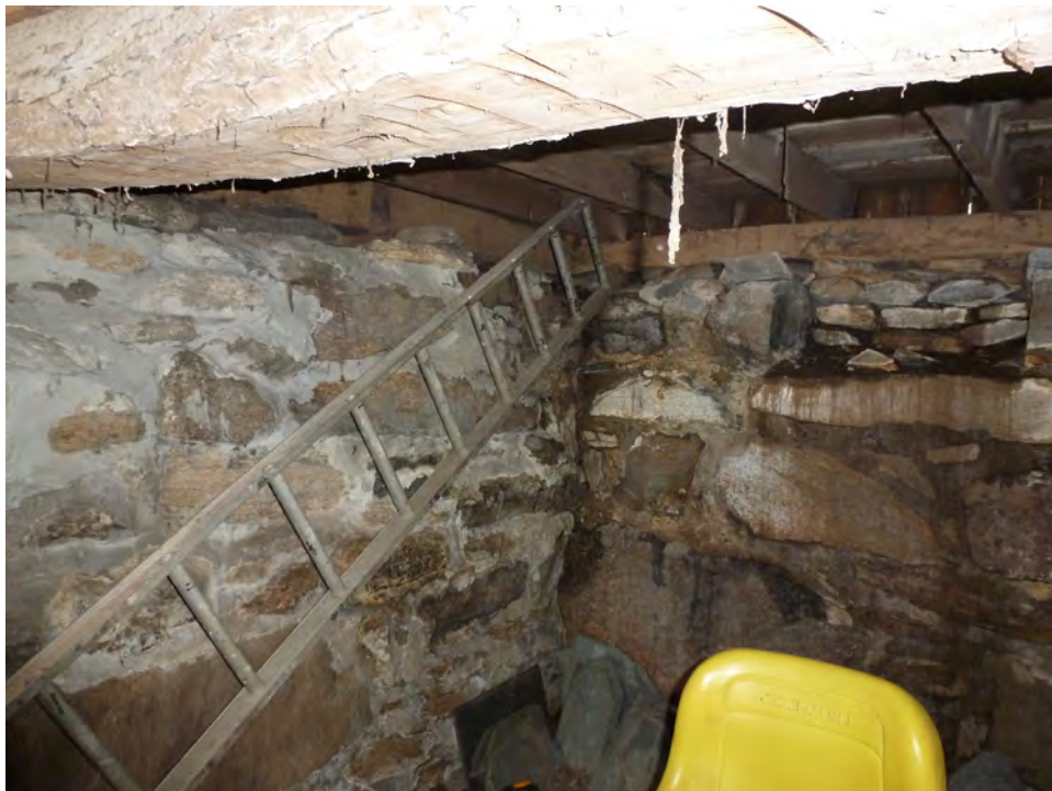
20. Interior view of the northwest corner of the basement. Note the mortared fieldstone walls. Camera facing northwest.
