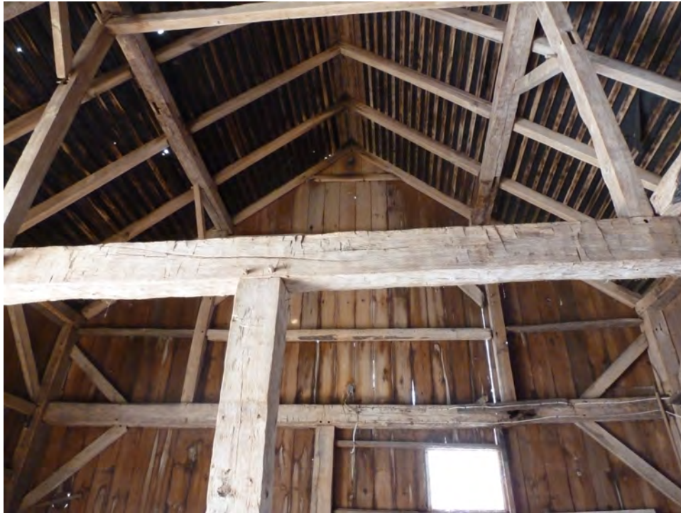
17. Interior view of the west gable-end of the Barn. Note the hand hewn marks on the timbers. Camera facing west.
