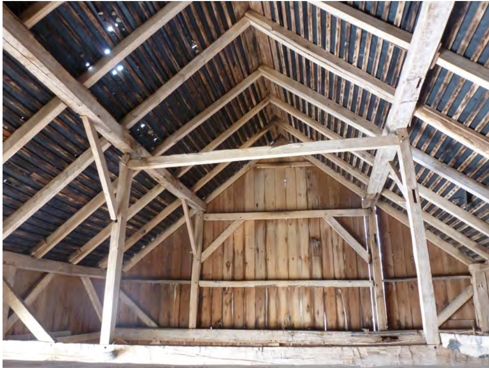
19. Interior view of the west gable-end of the Barn. Note the rafters meeting at the peak with no ridge-board and half-lap joints. Camera facing west.
