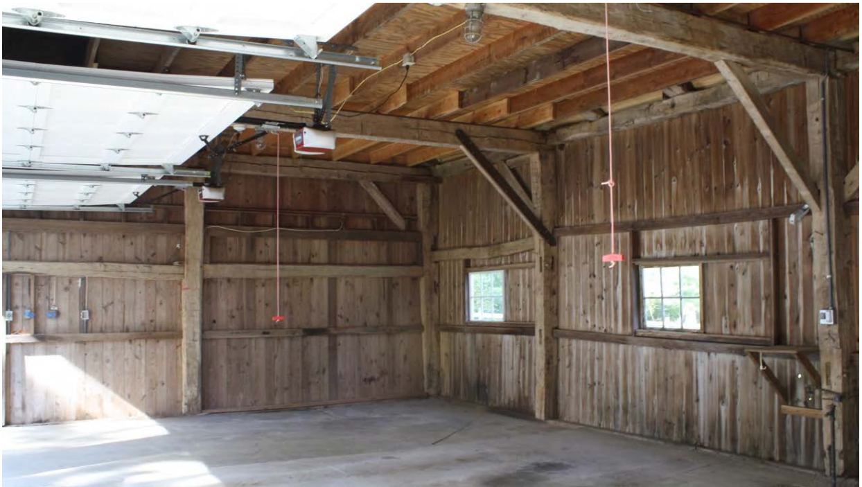
17. Interior of central block, camera facing northwest. Note gunstock posts and tie-girts at plate elevation.
